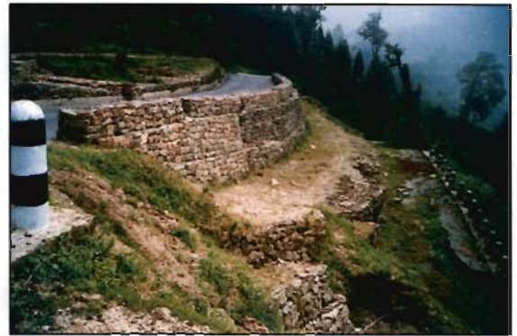
(f) Landslide and road sinking on Ghum-Sukhiapokhri road
