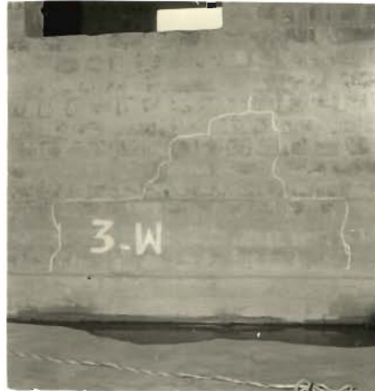
PHOTO 5.32_ LOCALISED INITIAL CRACKS IN WEST WALL (MODEL3)
