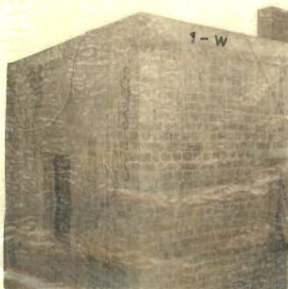
PHOTO 5.9 - CRACKS IN NORTH AND WEST WALLS (MODEL 1)
