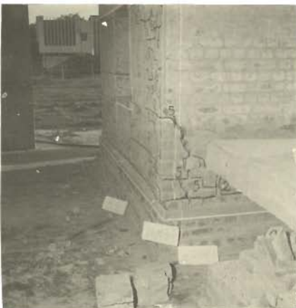
PHOTO 5.132 _ BOTTOM PORTION OF NORTH - EAST CORNER SHIFTED EASTWARD ( MODEL 8 )
