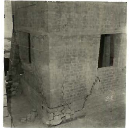
PHOTO 5.29_ SOUTH- WEST AND SOUTH-EAST CORNERS ACTING AS A SEPARATE STRUCTURAL ELEMENT ( MODEL 2 )
