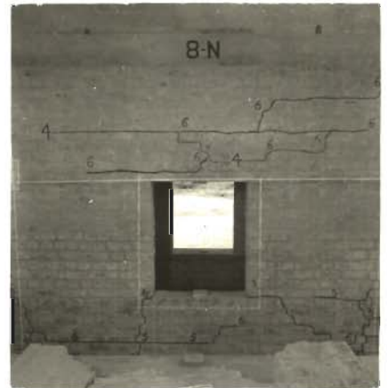
PHOTO 5.122_ WELL DISTRIBUTED CRACKS IN TOP AND BOTTOM SPANDEL S OF NORTH WALL ( MODEL 8 )
