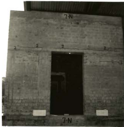
PHOTO 5.100 _ FEW FINE HORIZONTAL CRACKS IN NORTH SHEAR WALL ( MODEL 7 )
