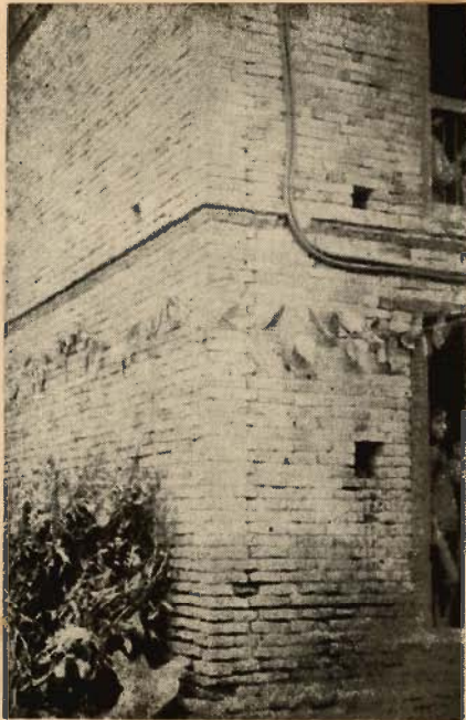
PHOTO 3.1 - BRICK BUILDING SHOWING USUAL TOOTHED JOINT AS SOURCE OF WEAKNESS DURING EARTHQUAKE (PHOTO BY A. S. ARYA)
