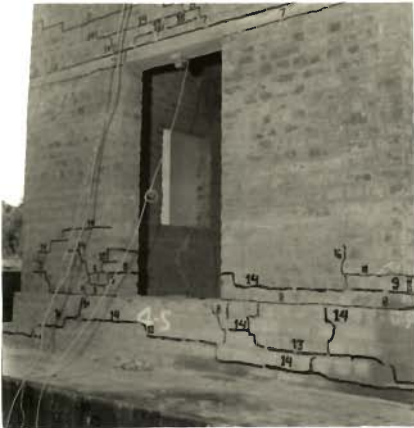
PHOTO 5-63-CRACKS IN BOTTOM REGION OF SOUTH WALL PIERS (MODEL 4)
