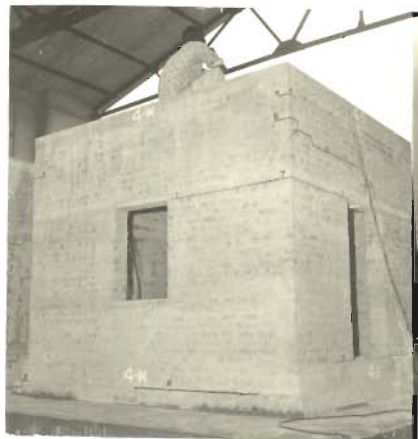
PHOTO 5.49_ FEW HORIZONTAL CRACKS IN WEST WALL (MODEL 4)
