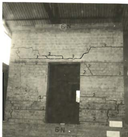
PHOTO 5-88-WELL DISTRIBUTED HORIZONTAL CRACKS IN NORTH SHEAR WALL (MODEL 6)
