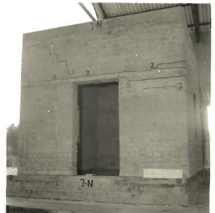
PHOTO 5.104 _ BOTTOM EDGES OF NORTH WALL PIERS LIFTED UP BY ABOUT 5mm, WEST WALL OVERHANGING OVER PLINTH BAND ( MODEL 7 )
