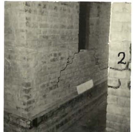
PHOTO 5.101 _ TWO REFERENCE LINES IN WHITE PAINT ON VERTICAL FACES OF PLINTH BAND TO MEASURE AMOUNT OF SLIDING ( MODEL 7 )
