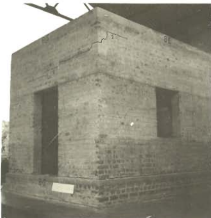
PHOTO 5.120 _ A HORIZONTAL CRACK AT JUNCTION OF, SOUTH AND EAST WALL WITH PLINTH BAND ( MODEL 8 )
