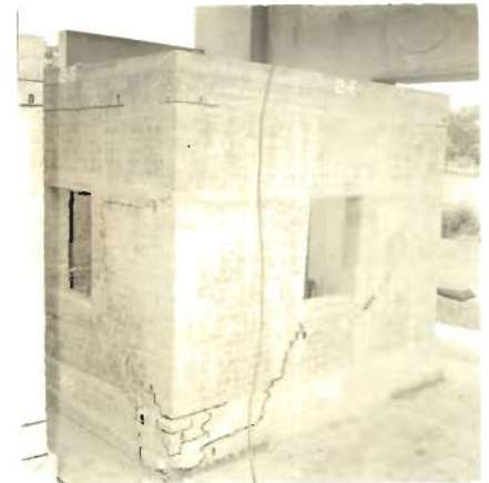
PHOTO 5.23_ CRACKS IN TOP SPANDREL OF EAST WALL (MODEL 2)
