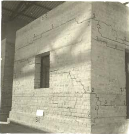
PHOTO 5.90 _ EXTENSIVE HORIZONTAL AND DIAGONAL CRACKS IN EAST WALL ( MODEL 6 )
