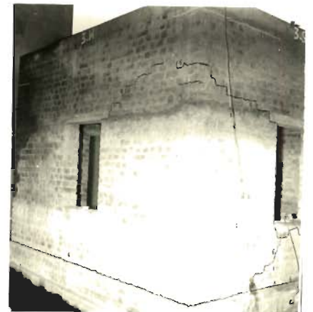
PHOTO 5.35_ HORIZONTAL CRACKS IN SOUTH AND WEST WALLS AT PLINTH LEVEL ( MODEL 3 )
