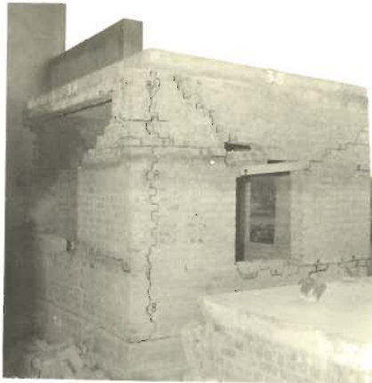
PHOTO 5.46_ SOUTH-SHEAR WALL IN BAD SHAPE (MODEL 3)
