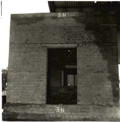
PHOTO 5.37_ HORIZONTAL CRACKS IN NORTH SHEAR - WALL (MODEL3)
