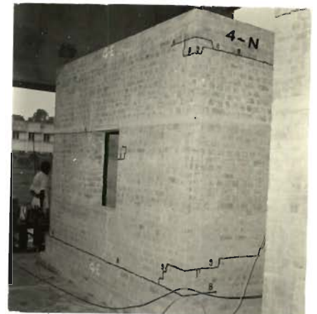
PHOTO 5.50_ CRACKS IN EAST CROSS-WALL (MODEL 4)
