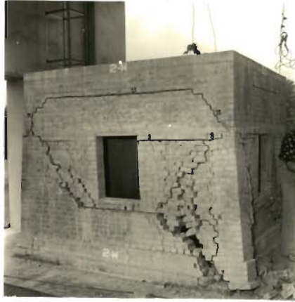
PHOTO 5.28 _ SOUTH-WEST CORNER PORTION ACTING AS A SEPARATE STRUCTURAL ELEMENT ( MODEL 2 )
