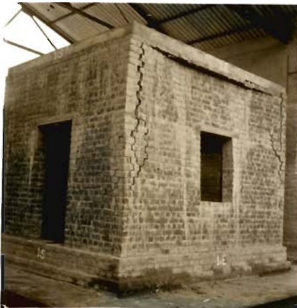
PHOTO 5.12 _ EAST CROSS- WALL DEFLECTED INWARD AT TOP (MODEL 1)
