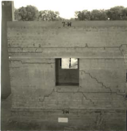
PHOTO 5.108_ A FEW HORIZONTAL AND DIAGONAL CRACKS IN WEST CROSS-WALL DURING SHOCK NO.6 (MODEL 7)
