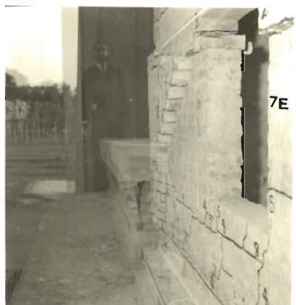
PHOTO 5.115 _ UPPER PORTION OF LEFT PIER OF EAST WALL THROWN OUT DURING SHOCK NO.8 (MODEL 7)
