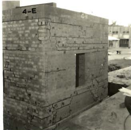
PHOTO 5-64-NORTH-EAST AND NORTH WEST CORNERS PUSHED OUTWARD (MODEL 4)
