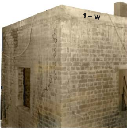
PHOTO 5.9 _CRACKS IN NORTH AND WEST WALLS (MODEL 1)
