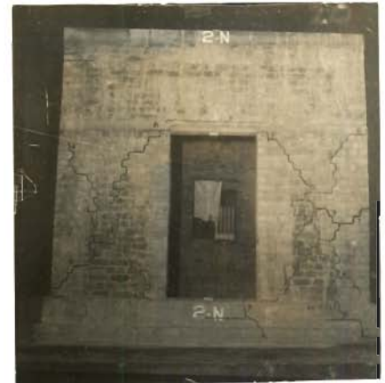
PHOTO 5.20_ MOSTLY DIAGONAL CRACKS IN NORTH WALL (MODEL 2)
