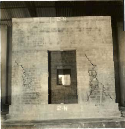
PHOTO 5.18_ DIAGONAL CRACKS IN NORTH SHEAR WALL (MODEL 2)
