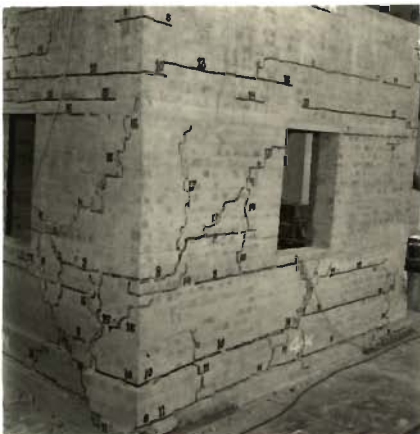
PHOTO 5-66-RIGHT PORTION OF WEST WALL BETWEEN PLINTH AND WINDOW SILL LEVELS SHIFTED OUTWARDS (MODEL 4)
