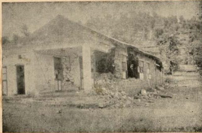
PHOTO 2.1_ DAMAGE TO SCHOOL IN KOYNA EARTHQUAKE, INDIA ( STAR CRACK PATTERN IN BRICK WALL )
