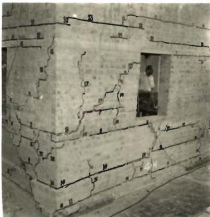
PHOTO 5-69-PORTION BETWEEN PLINTH AND WINDOW SILL LEVELS OF WEST WALL SHIFTED TOWARDS SOUTH (MODEL 4)
