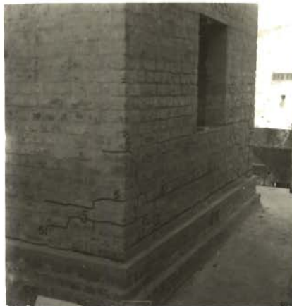
PHOTO 5.121_ MANY CRACKS IN BOTTOM SPANDEL OF NORTH SHEAR WALL ( MODEL 8 )
