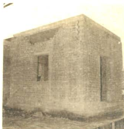
PHOTO 5.14 - TOP PORTION OF WEST WALL FELL DOWN (MODEL 1)
