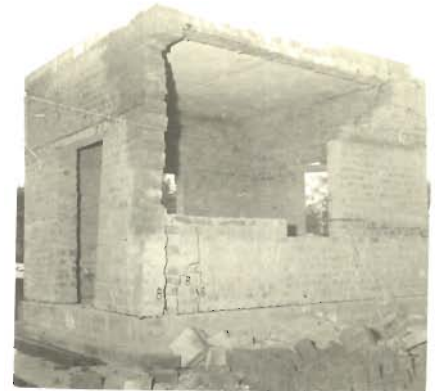
PHOTO 5.47_ LARGE CHUNK OF MASONRY FROM WEST WALL FELL DOWN (MODEL 3)
