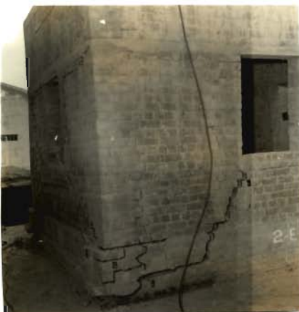
PHOTO 5.24_ BOTTOM PORTION OF SOUTH - WEST CORNER PUSHED OUTWARDS (MODEL 2)
