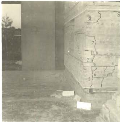
PHOTO 5.118 _ UPPER PART OF WEST WALL RIGHT PIER DISPLACED OUTWARD TOWARD NORTH ( MODEL 7 )
