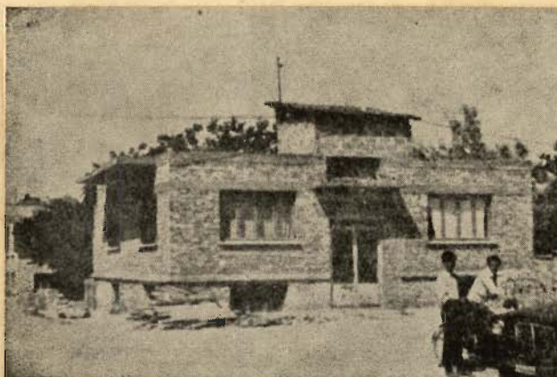
Photo 1.1 BRICK BUILDING WITH R.C. BANDS SHOWING EFFECTIVENESS OF THE BAND IN KEEPING THE BUILDING SAFE IN AREA OF MOST SEVERE SHAKING IN EARTHQUAKE OF MAY 1971 (TURKEY)
