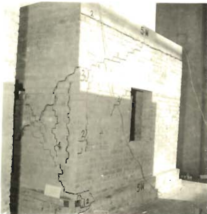
PHOTO 5-84-NORTH SHEAR WALL AT THE VERGE OF FALLING DOWN WHILE WEST WALL IN A BETTER SHAPE (MODEL 5)
