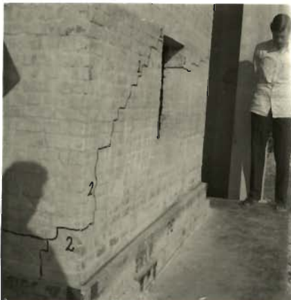
PHOTO 5.102 _ A BLACK STRIP SEEN AT PLINTH BAND AFTER SLIDING OF EAST WALL TOWARDS WEST ( MODEL 7 )
