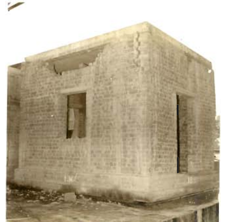
PHOTO 5.14 _ TOP PORTION OF WEST WALL FELL DOWN (MODEL 1)
