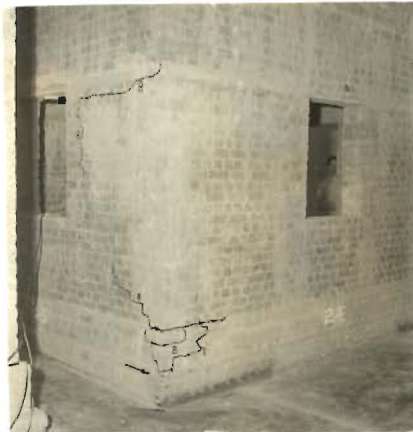
PHOTO 5.22_ EAST PIER OF SOUTH WALL WITH FEW CRACKS (MODEL 2)
