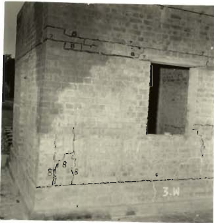
PHOTO 5.45_ WEST CROSS WALL BADLY DAMAGED (MODEL 3)
