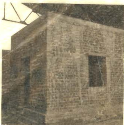
PHOTO 5.10 - VERTICAL CRACKS IN EAST CROSS WALL (MODEL 1)
