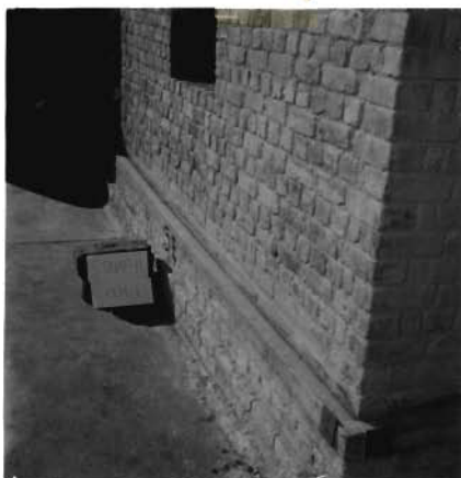
PHOTO 5.75_EAST WALL MOVED TOWARDS WEST (MODEL 5)
