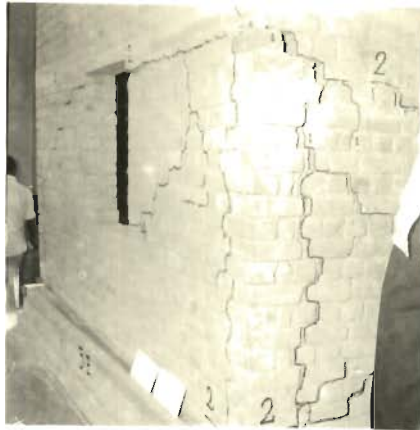
PHOTO 5-82-SLIDING OF SUPER - STRUCTURE SEEN AT PLINTH BAND OF EAST WALL (MODEL 5)
