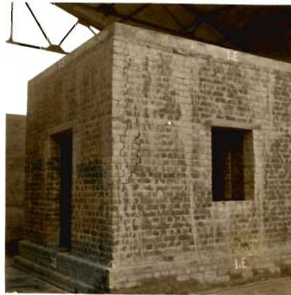
PHOTO 5.10 _VERTICAL CRACKS IN EAST CROSS WALL (MODEL 1)
