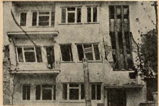
PHOTO 3.2 - SHEAR STRUCTURE BEHAVIOUR OF A THREE STOREYED BRICK BUILDING SUBJECTED TO GEDIZ EARTHQUAKE OF 1970 (TURKEY)
