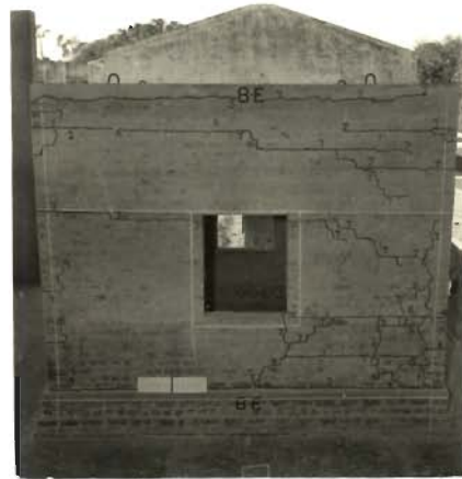
PHOTO 5.130 _ RIGHT PIER OF EAST CROSS WALL HEAVILY DAMAGED ( MODEL 8 )
