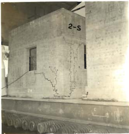
PHOTO 5.21_ CRACKS IN WEST PIER OF SOUTH WALL AND WEST WALL (MODEL 2)
