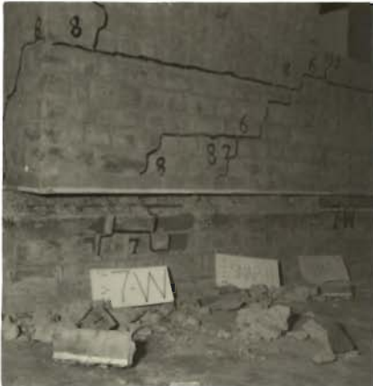
PHOTO 5.117_ FOUNDATION MASONRY UNDER WEST WALL VERY BADLY DAMAGED ( MODEL 7 )
