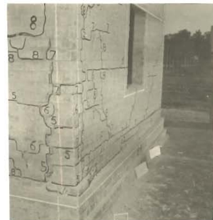
PHOTO 5.133 _ NORTH WEST CORNER DISPLACED WESTWARD AT PLINTH BAND BY 30 mm ( MODEL 8 )
