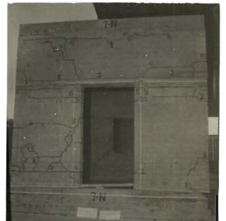
PHOTO 5.113 _ SEVERLY DAMAGED NORTH SHEAR WALL DURING SHOCK NO.8 (MODEL 7)
