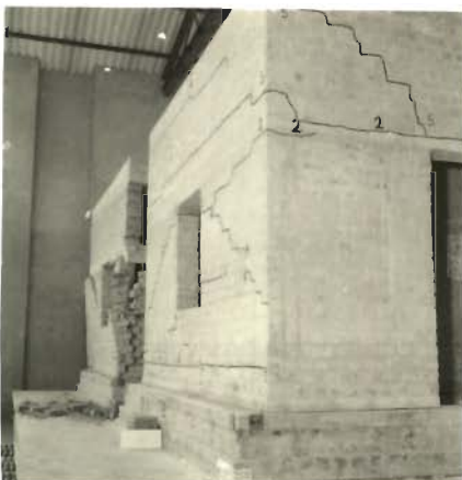
PHOTO 5.105 _ LARGE SHIFT OF EAST WALL AT PLINTH BAND ( MODEL 7 )
