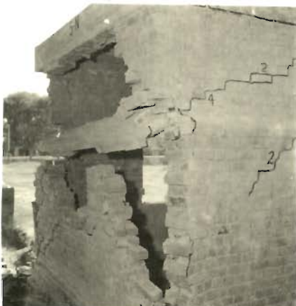
PHOTO 5-87-MAJOR PORTION OF NORTH SHEAR WALL COLLAPSED (MODEL 5)
