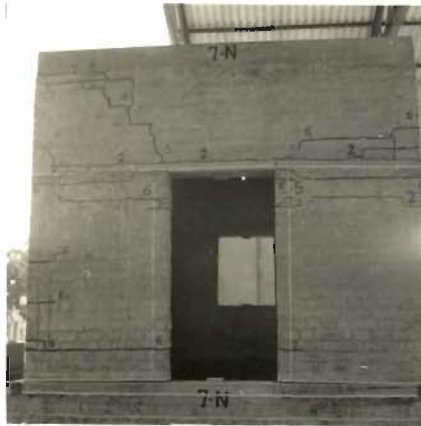
PHOTO 5.109_ MAINLY HORIZONTAL AND FEW DIAGONAL CRACKS IN NORTH SHEAR WALL DURING SHOCK NO.6 (MODEL 7)
