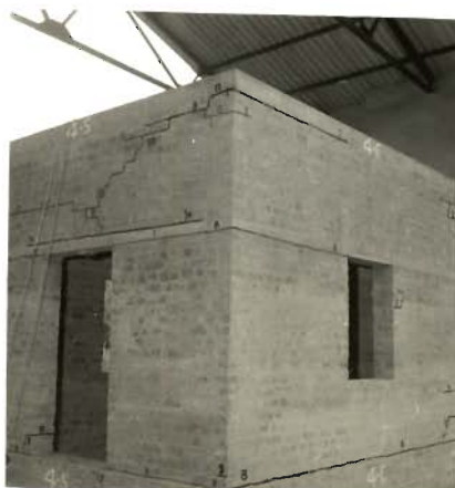
PHOTO 5.53_ SIGNIFICANT HORIZONTAL AND DIAGONAL CRACKS IN TOP SPANDREL OF SOUTH WALL (MODEL 4)
