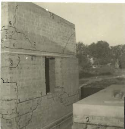
PHOTO 5.114 _ RIGHT PIER SEPARATED FROM RIGHT PORTION OF BOTTOM SPANDREL OF SOUTH WALL (MODEL7)
