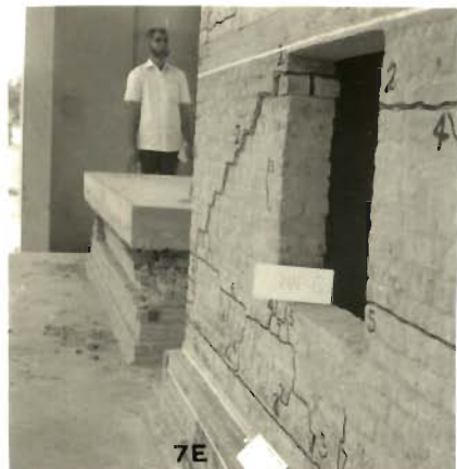
PHOTO 5.112_ LEFT PIER OF EAST WALL SEPARATED INTO TWO PORTIONS, WESTWARD SLIDING OF WALL (MODEL 7)
