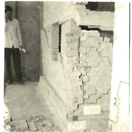
PHOTO 5-86-EAST CROSS-WALL IN VERY BAD SHAPE (MODEL 5)
