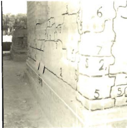
PHOTO 5.127 _ BOTTOM REGION OF NORTH - WEST CORNER BADLY DAMAGED ( MODEL 8 )
