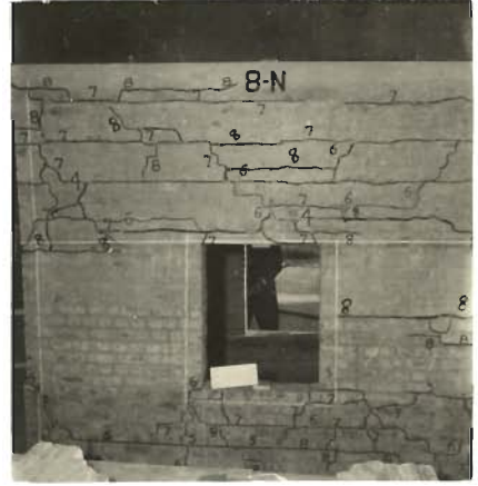
PHOTO 5.131 _ SEVERLY DAMAGED NORTH WALL DURING SHOCK NO.8 (MODEL 8 )
