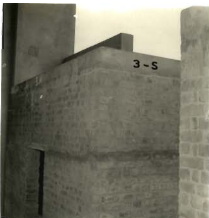
PHOTO 5.33_ INITIAL CRACKS BELOW ROOF SLAB OF SOUTH WALL ( MODEL 3 )
