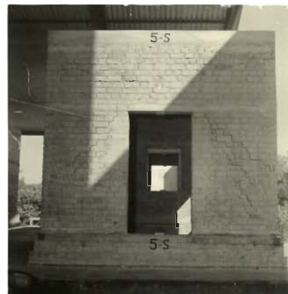
PHOTO 5.74_DIAGONAL CRACKS IN BOTH PIERS OF SOUTH SHEAR WALL (MODEL 5)
