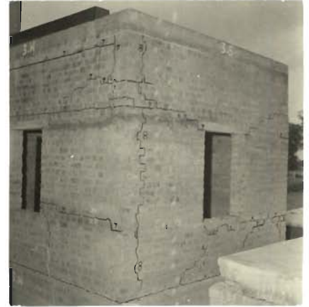
PHOTO 5.41_ A SIGNIFICANT VERTICAL CRACK NEAR SOUTH - WEST CORNER ( MODEL 3 )
