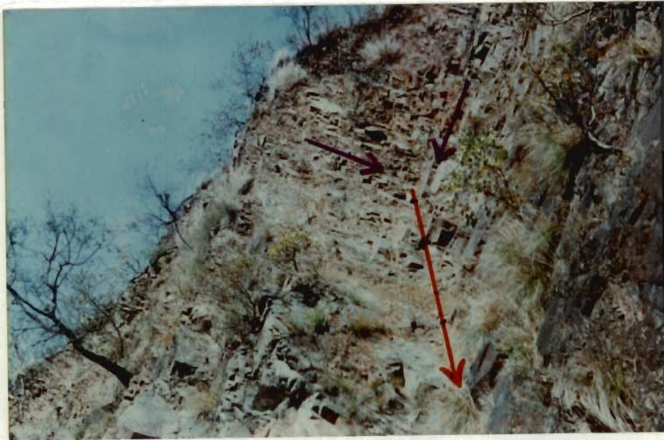
Plate 3.3 Wedge failure in metavolcanic
