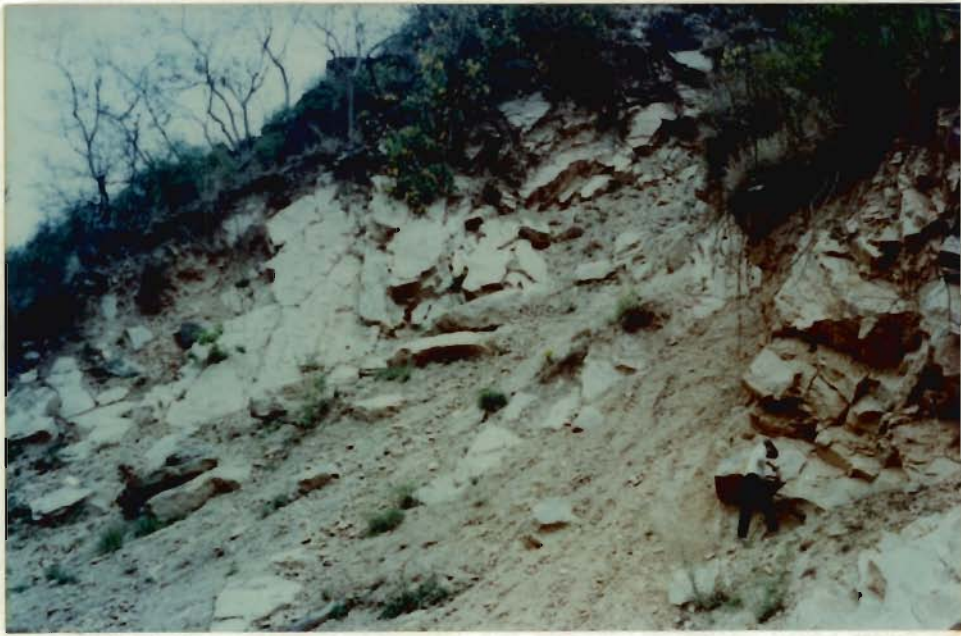
Plate 3.1 Planar failure in quartzite
