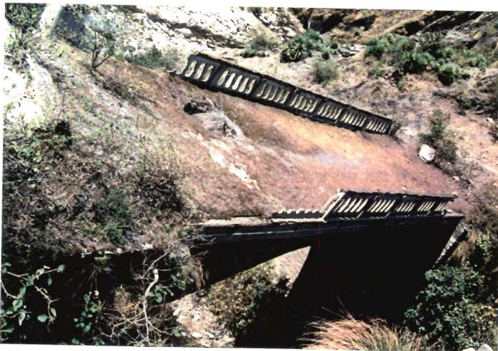
A rock block, fall from the adjoining slope, damaged a bridge between Tehri and Bhaldiyana.
