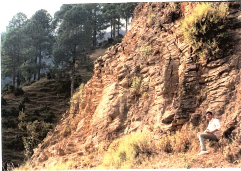
Failure along axial plane cleavage joints in an asymmetric antiform in phyllites south of Surkunda.
