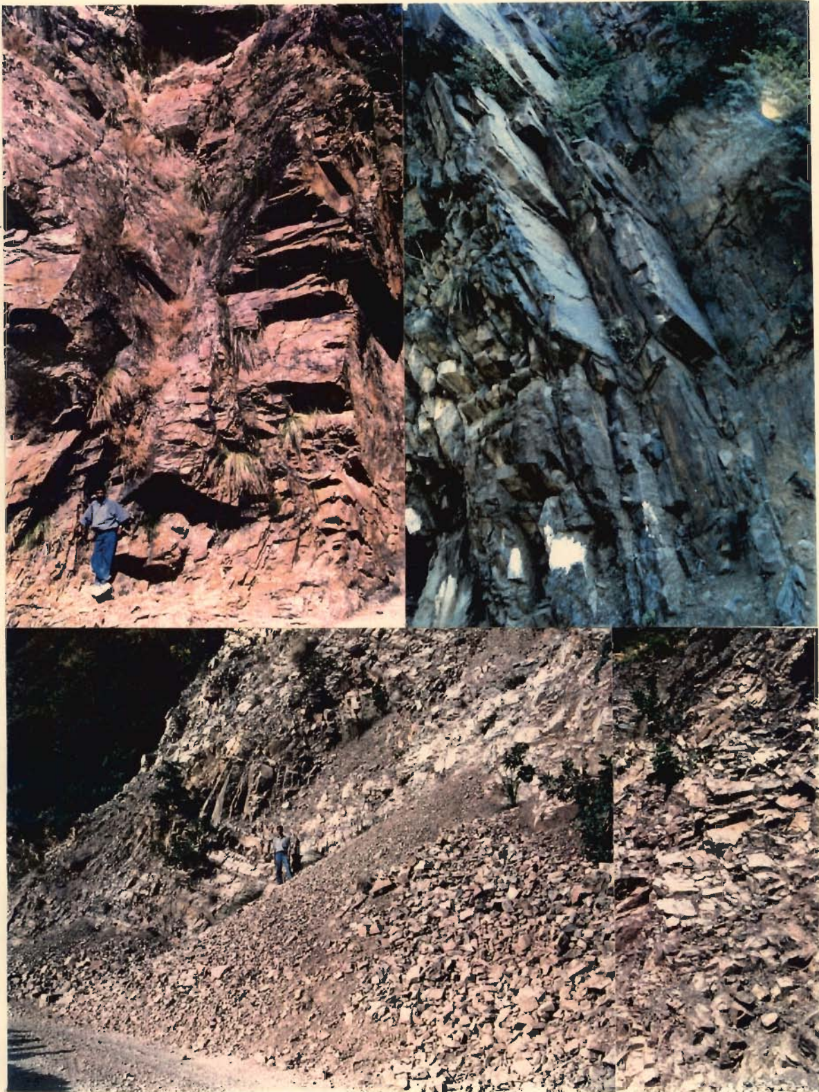
PLATE 5.4 WEDGE MODE OF FAILURES IN RESERVOIR AREA
