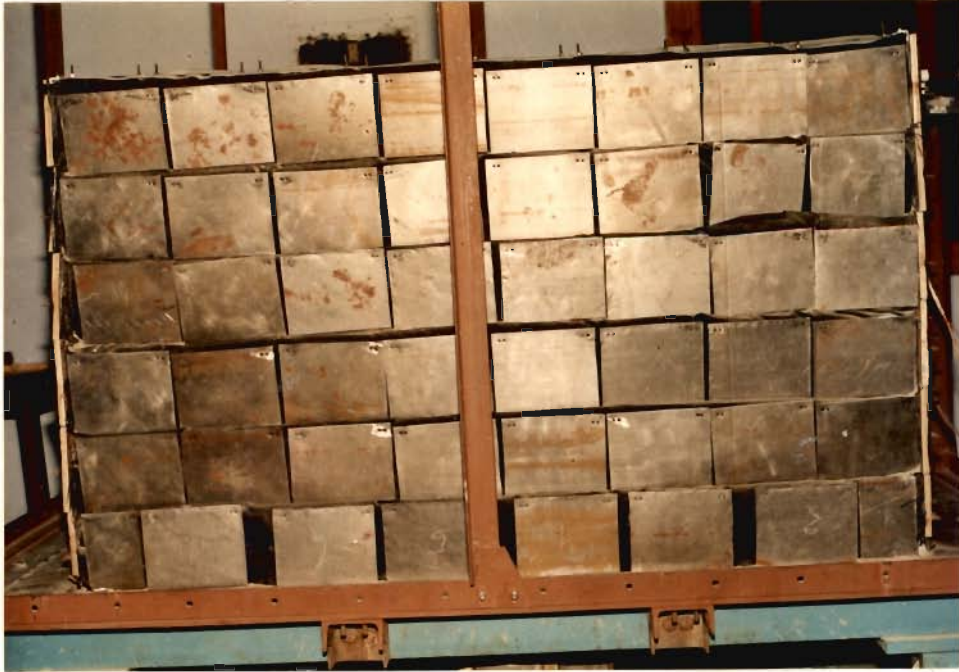
FIG. 4. 4. 3 VIEW OF THE TRANSVERSE FACE OF RE- TEST EMBANKMENT AT THE END OF CONSTRUCTION AFTER REMOVAL OF FORMWORK.
