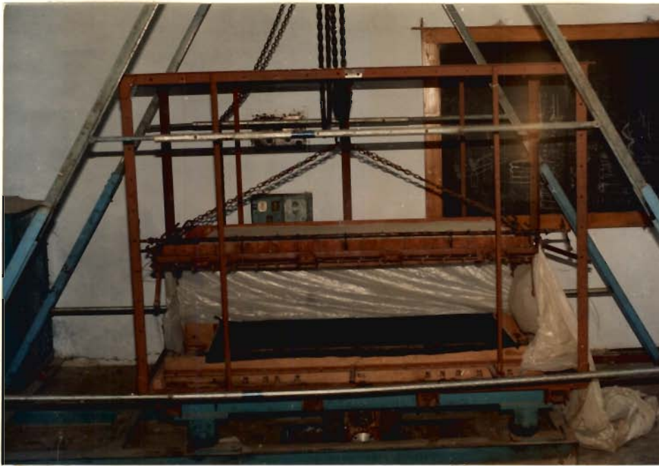
FIG. 4.4.9 VIEW OF THE SETUP AT THE BEGINNING OF PREPARATION OF RE TEST EMBANKMENT.
