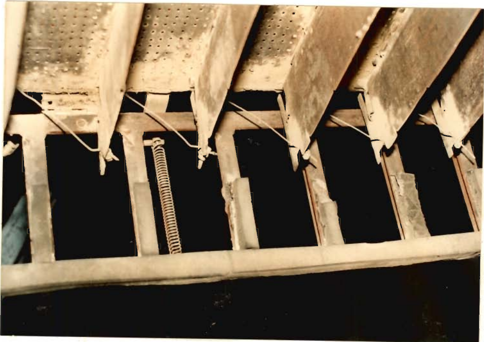
FIG.3.2.6 CLOSE VIEW OF SRA WITH SHUTTERS IN THEIR OPEN POSITION.
