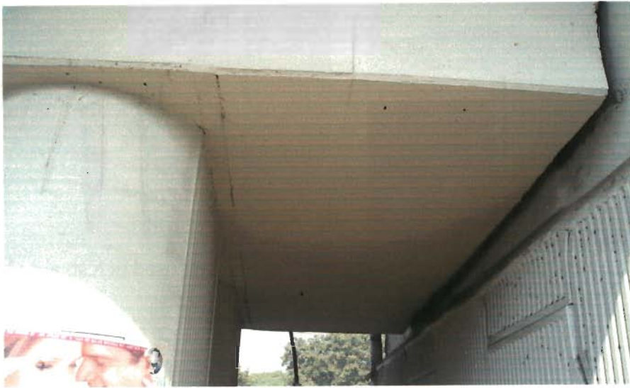
Fig. 1.5: Deck extension integral flyover built in New Delhi, piers integral with superstructure and expansion joint near abutment backwall
