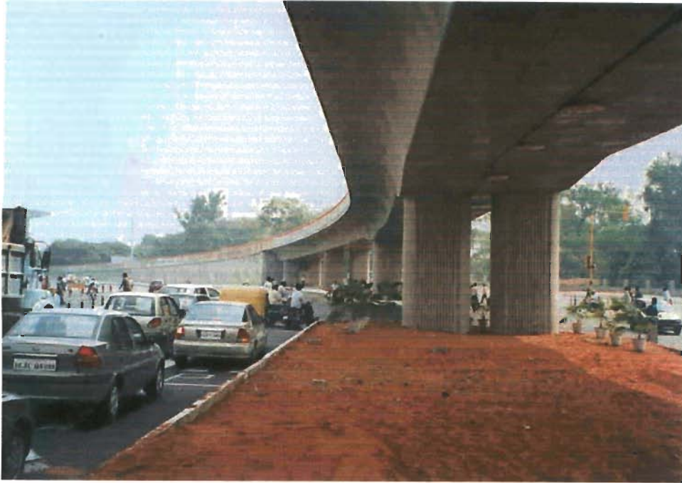
Fig. 1.10: Integral flyover with RC voided slab in Kalkaji flyover, New Delhi, India
