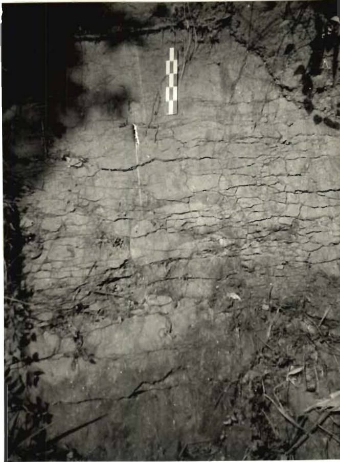
Figure 4.15. Field photograph showing southward dipping (facing the viewer) fault in soil. The slip surface also show northward dipping cracks. Loc.-10 km north of Dauki towards Pynursla.
