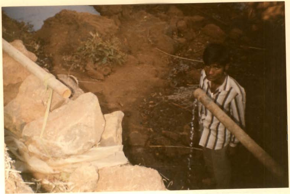
Fig.4.14 : Breaking-apart of the pipe-lines tapping spring water in the hilly tracts (Dhangarvadi-Spring No.33) (elevation 975m above MSL).
