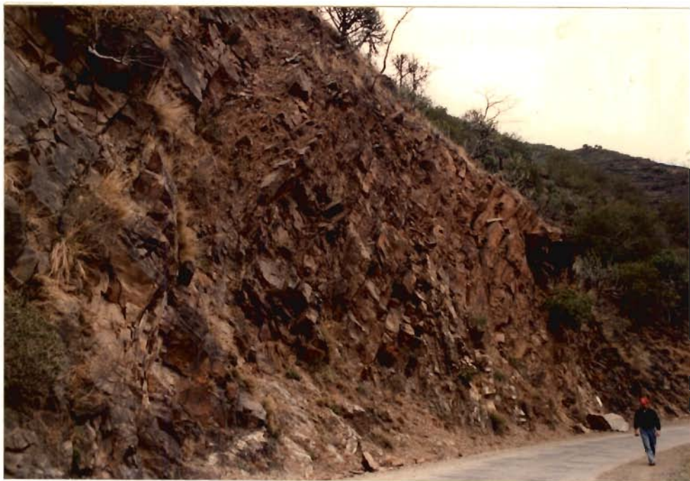
Fig. 3.12 : Rock fall from Over Hanging Scar Face of the Quartzite (52 km from Rishikesh)
