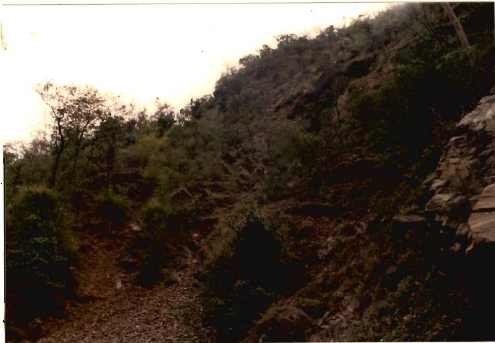
Fig. 5.5 : Large Planar Failure in Well Jointed Quartzite (38.5 km from Rishikesh)
