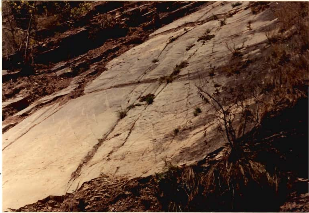
Fig. 3.11 : Rock Slide on Dip-Slopes of Quartzite Caused by Toe Excavation (32 km from Rishikesh)
