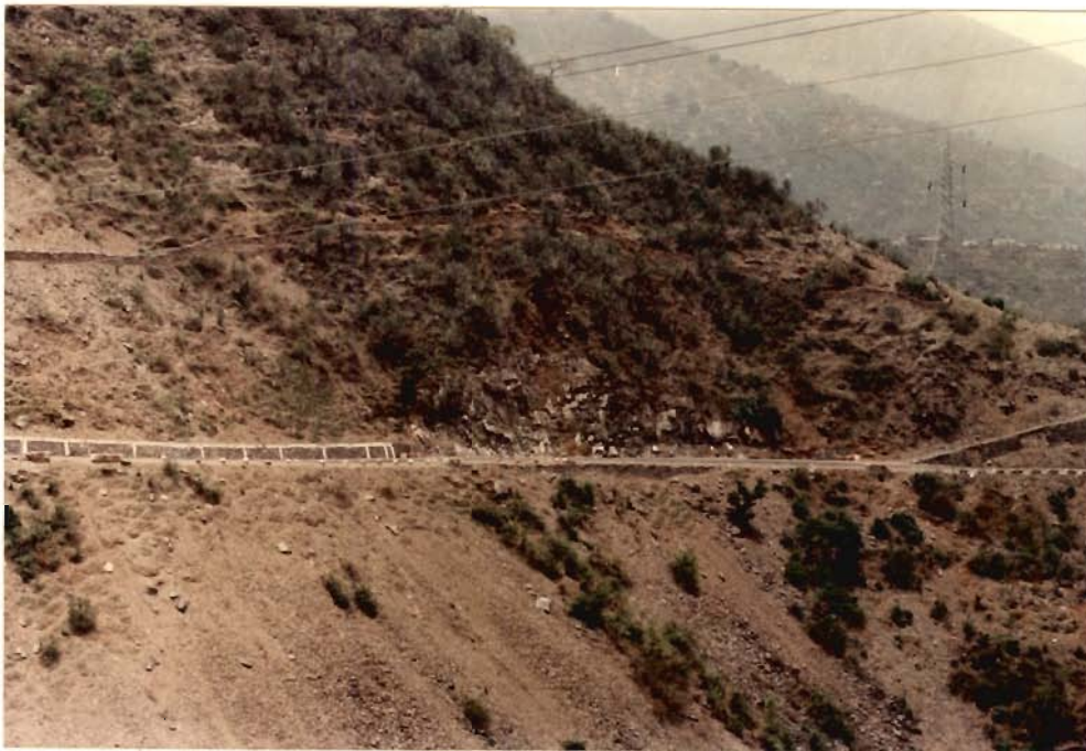
Fig. 5.10 : Wedge Failure in Well Jointed Quartzite (52.8 km from Rishikesh)
