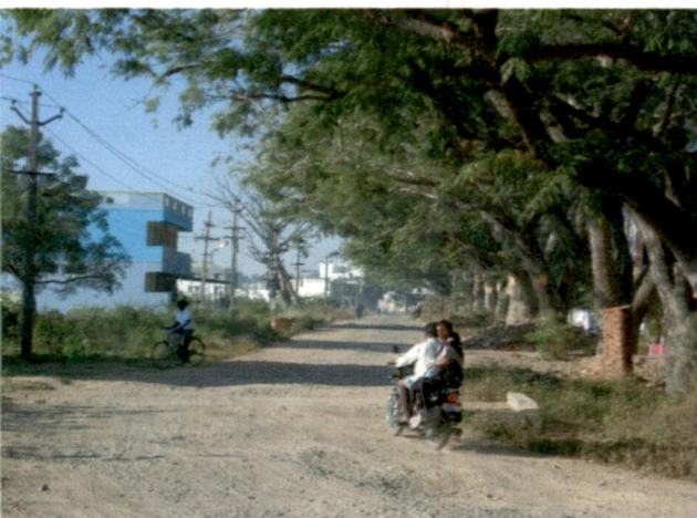
Fig 6.37: Bad Road Surface
