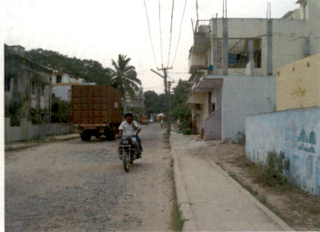
Fig 6.32: Sidewalks Not Maintained
