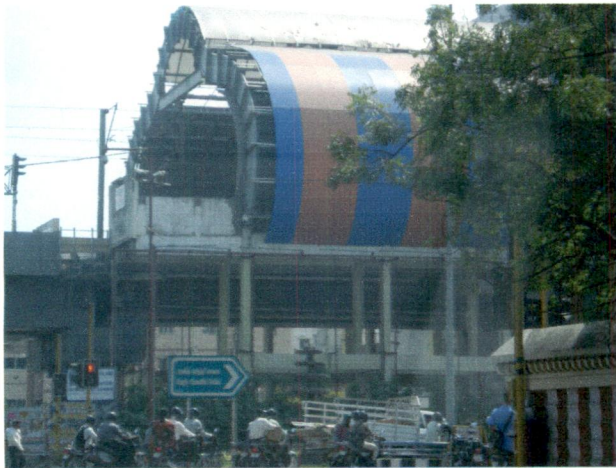
Fig 5.5: Entry to Rajiv Gandhi Salai at Madhya Kailash Junction. Kasturibai Nagar Metro Station.
