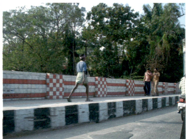
Fig.4.4: Raised Pedestrian Foot Path Making It Difficult To Climb For Elderly, Children And Physically Challenged.
