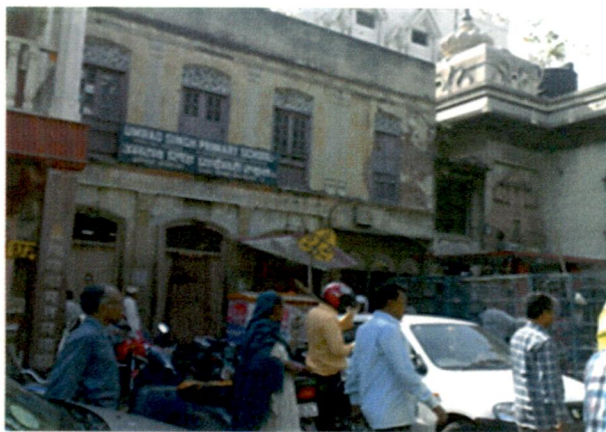
Fig 3.4: Deterioration of Structures
