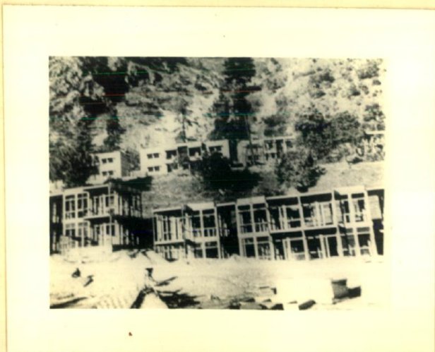
FOREGROUND SHOWS DOUBLE STOREY FRAME WORK READY FOR LATHPLASTER/ HOLLOW BLOCK MASONRY. NOTICE THAT THE FRAME WORK APPEARS LIKE MATCHTICK HENCE THE NAME OF "MATCHTICK DESIGN OF PREPABRICATED CONSTRUCTION".
