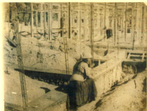
PLINTH BEAM CASTING COMPLETED. PLINTH OF GROUND FLOOR CAN BE SEEN ERECTED AT FAR END.
