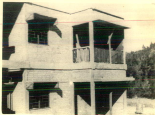
21 VIEW SHOWING WALL PANELS COMPLETED WITH INFILL MATERIAL OF CEMENT HOLLOW BLOCKS. WINDOW/VERANDAH CHAJJAS CAST-IN-SITU CAN ALSO BE SEEN.
