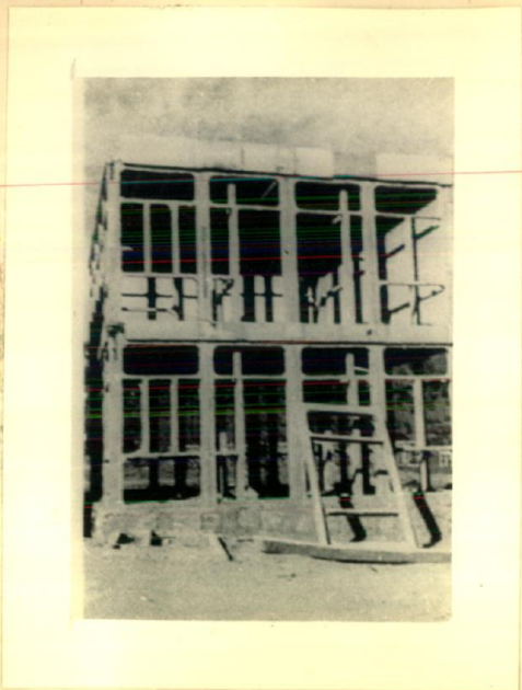
FIRST FLOOR PANELS AND COLLAR BEAMS ERECTED AND ALL CAST-IN-SITU WORK COMPLETED
