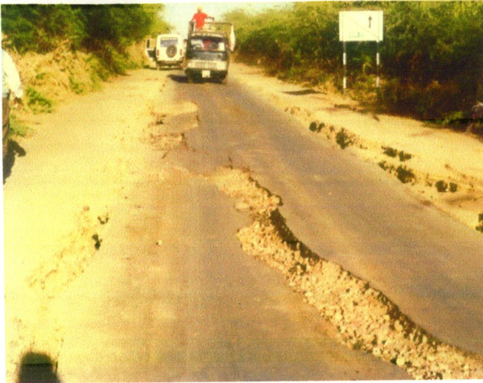
Fig. 2.8 Damage to Highway Pavement near Rapar due to Lateral Spreading of Soil (EERI Special Earthquake Report, 2001)
