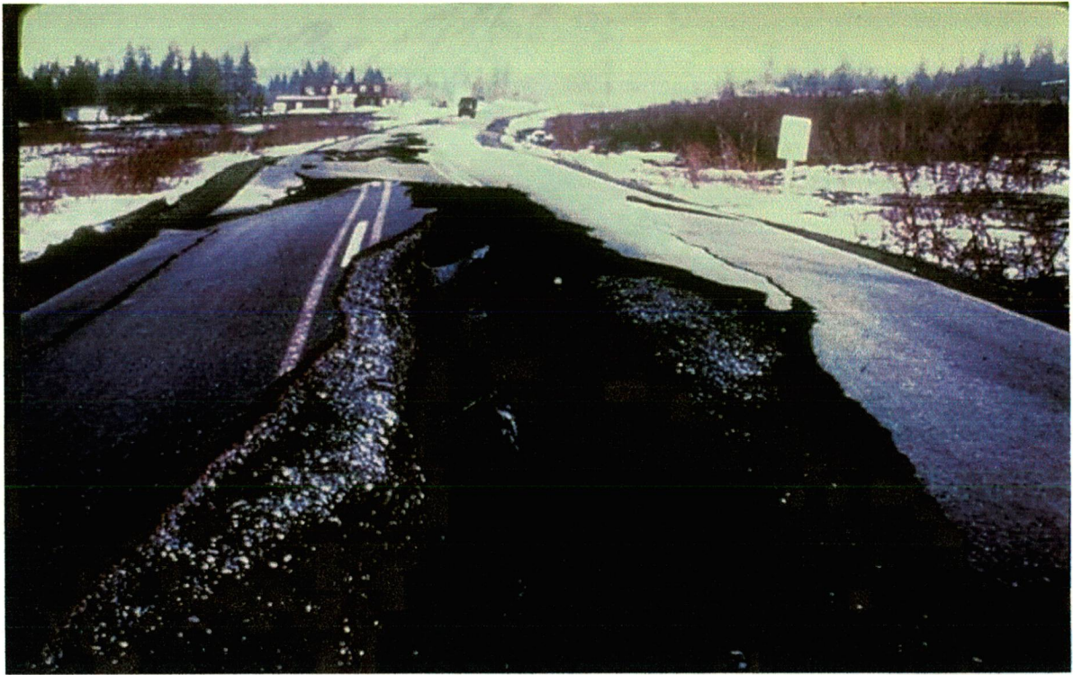
Fig. 2.3 Fissured Highway Embankment, 1964 Alaska Earthquake
