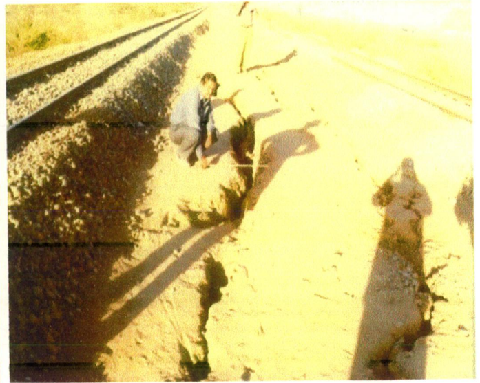
Fig. 2.9 Rail Embankment at Vaka Nala (EERI Special Earthquake Report, 2001)
