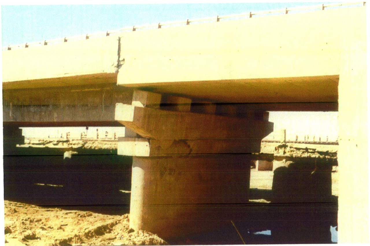
Fig. 2.10 Damage to the Unequal-height Bed Blocks at RC Bridge near Vondh (EERI Special Earthquake Report, 2001)
