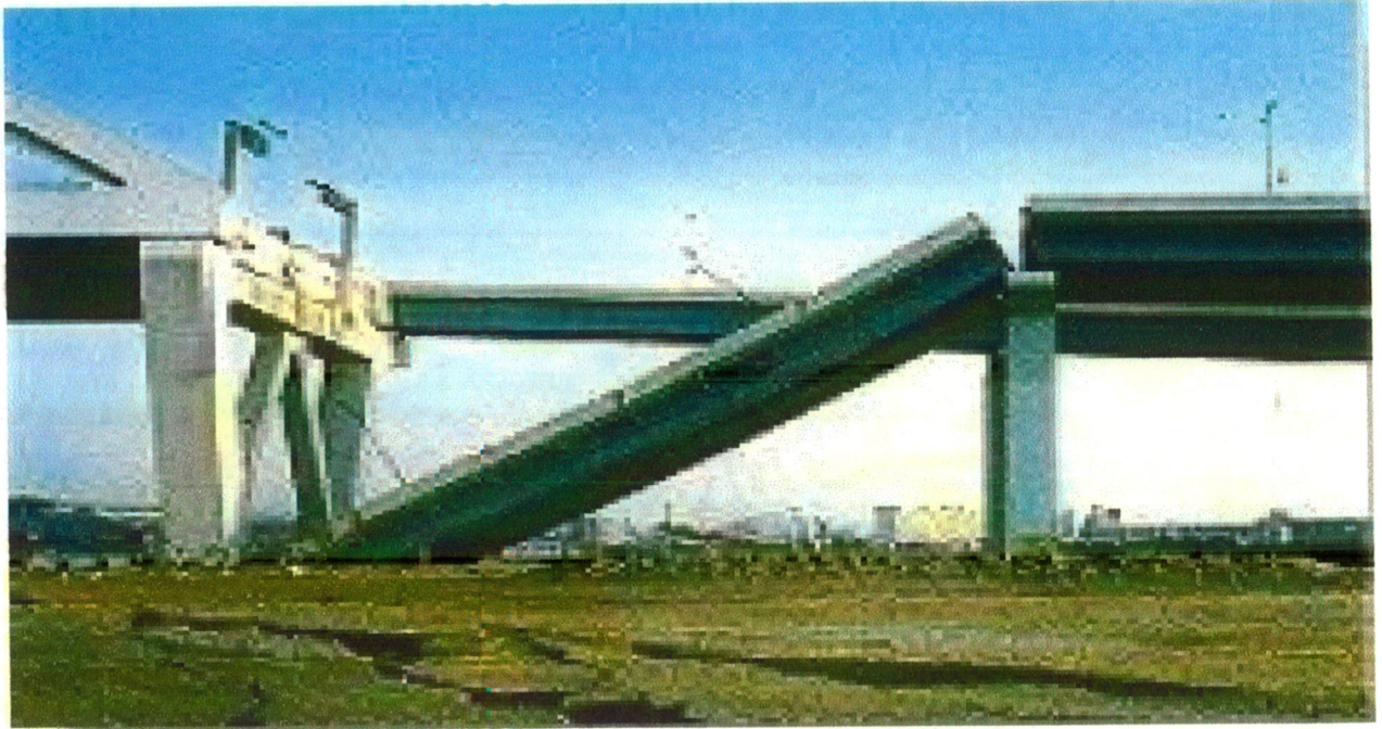
Fig. 2.7 Fallen Bridge Deck, 1995 Kobe Earthquake ( www.ce.Washington.edu/liquefaction/html/main.html )
