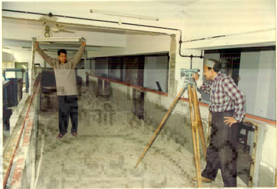
Plate 3.1: SHOWING LEVELLING PROCEDURE OF RAILS AND TROLLEY AT THE LAST STAGE OF FLUME CONSTRUCTION.
