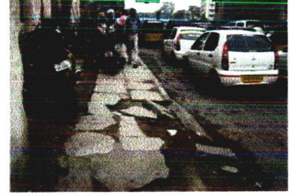
Fig. 5.43: Broken sidewalks Nungambakkam Source: By Author
