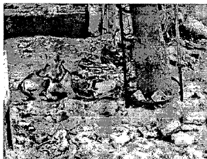
Fig. 4.29: Sidewalk with debris, Noida
