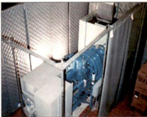
Figure 5.28: Sound Curtain for Lift Machine Room
