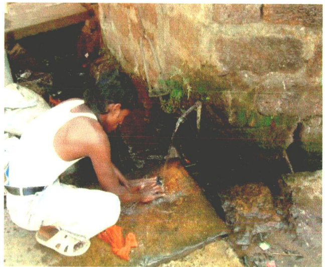
Figure 5.16: A water standpipe in poor condition Source: Primary survey by author
