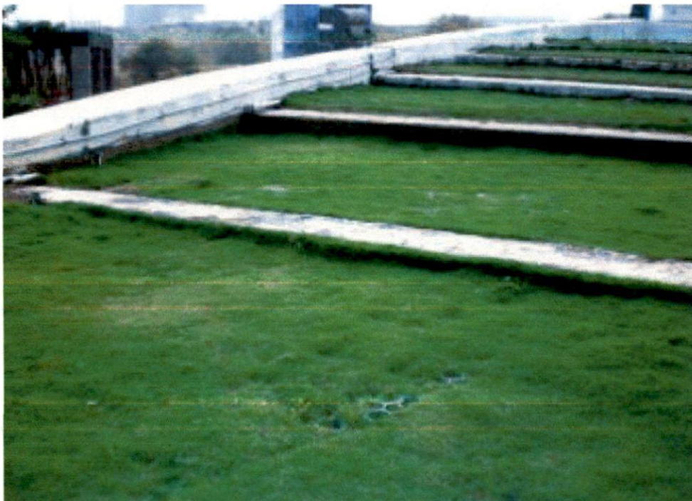
Figure3.10. This section of the CII green roof reveals a section of structural pavers where the sod is thinned, likely a seam.
