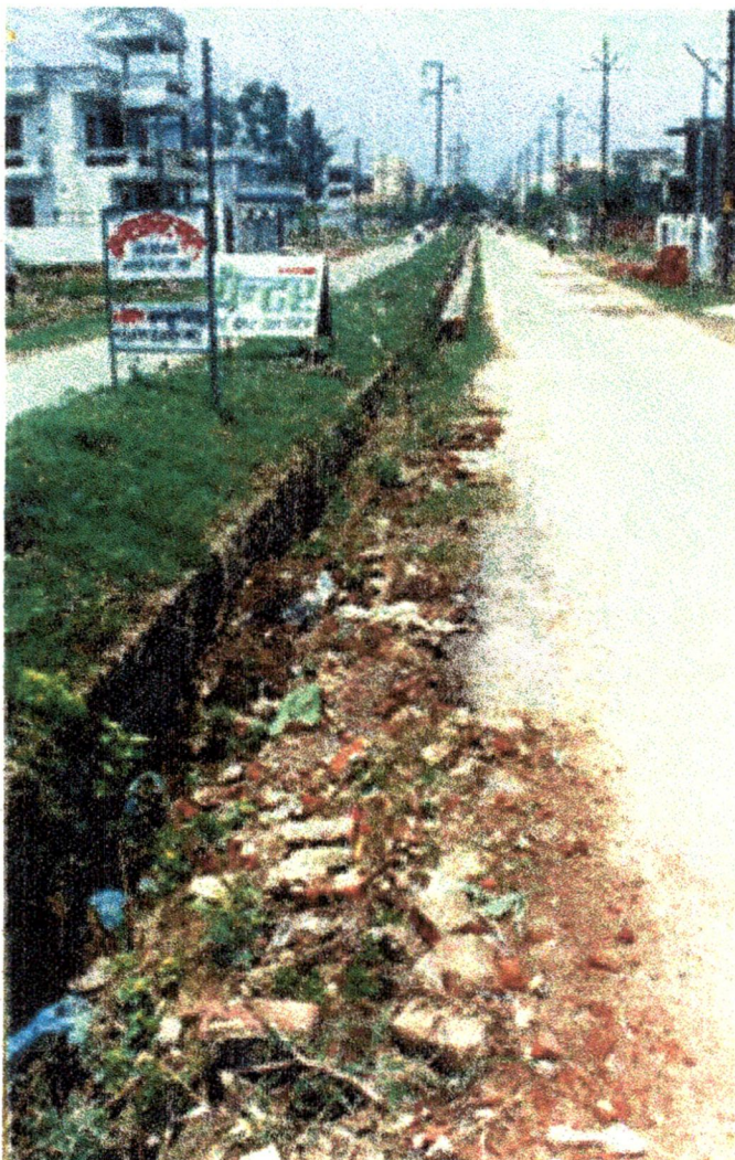
Poor drainage conditions
