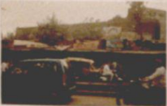
SOUTHERN SIDE OF RAMBAGH GATE WITH WALL STRUCTURAL DETERIORATION.
