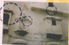
BUILDINGS NEED URGENT RESTORATION & CONSOLIDATION. • PIGEONS ARE SERIOUS THREAT. • ACCUMULATION OF MOISTURE IS A SERIOUS PROBLEM FOR STRUCTURE.
