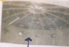
WOODEN STRUCTURES IN GARDEN NEED IMMEDIATE MEASURES FOR PRESERVATION.
