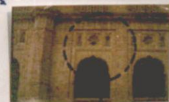
BROKEN JALLIES NEGLECT HERITAGE.
