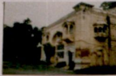
MONUMENTS OF RAMBAGH. • NEGLECTED • USED AS CLIMB • ADDITIONS, ALTERATIONS, REPAIRS NOT HARMONISING WITH ORIGINAL FABRIC.
