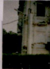
• RAIN WATER / SEWER PIPES & ELECTRIC CABLES SPOILING THE CHARACTER
