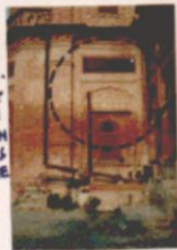
LACK OF MAINTENANCE.
