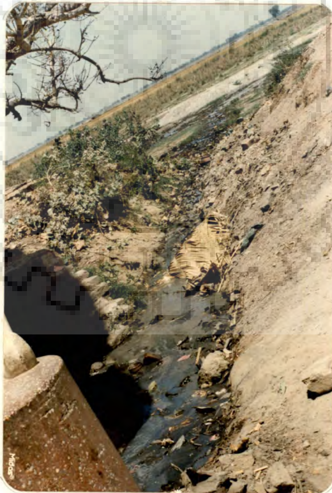
EFFLUENT MOVING TOWARDS GANGA AT RAJGHAT NARORA PLATE-6
