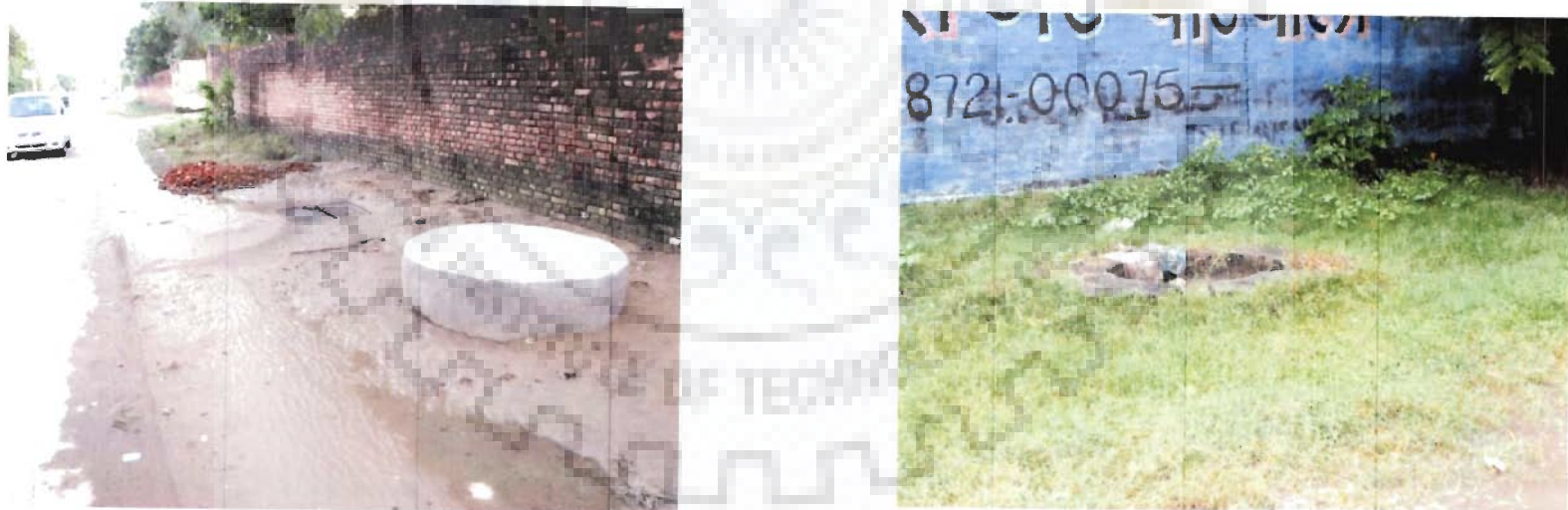
Fig 5.45: Rain Water Harvesting Structures Installed On Experimental Basis under State Of Neglect and Have Become Redundant
