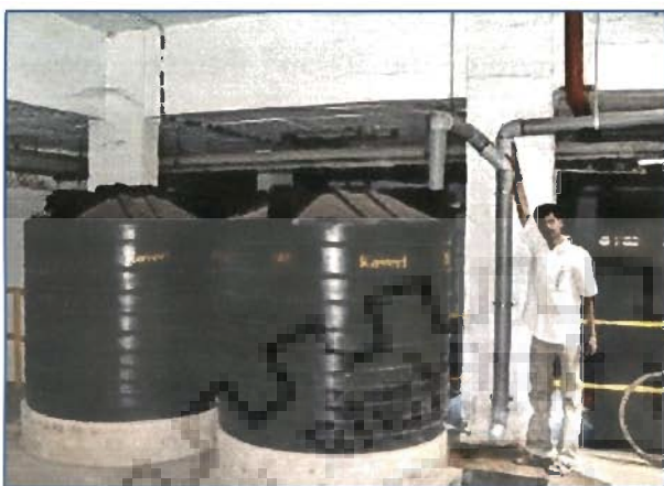
Figure 3.4 Simple rainwater harvesting tank in apartment, (Source: www.rainwaterclub.org )
