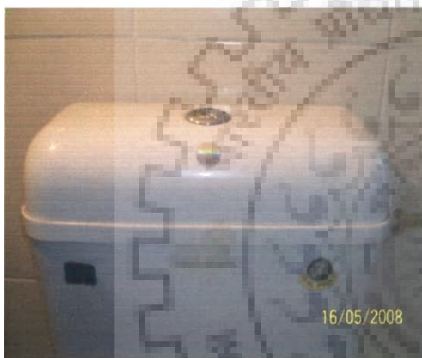
Figure 3.11 Dual flush cisterns
