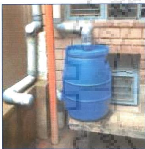
Figure 3.2 PVC Drum filters
