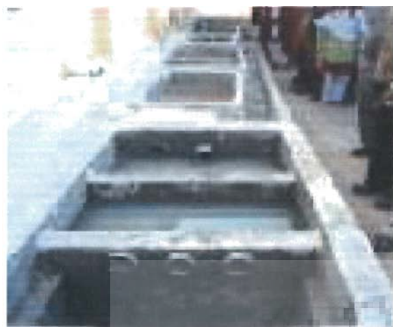
Figure 4.8 Settling tank for primary treatment of grey water in school in MP (NEERI, 2007)
