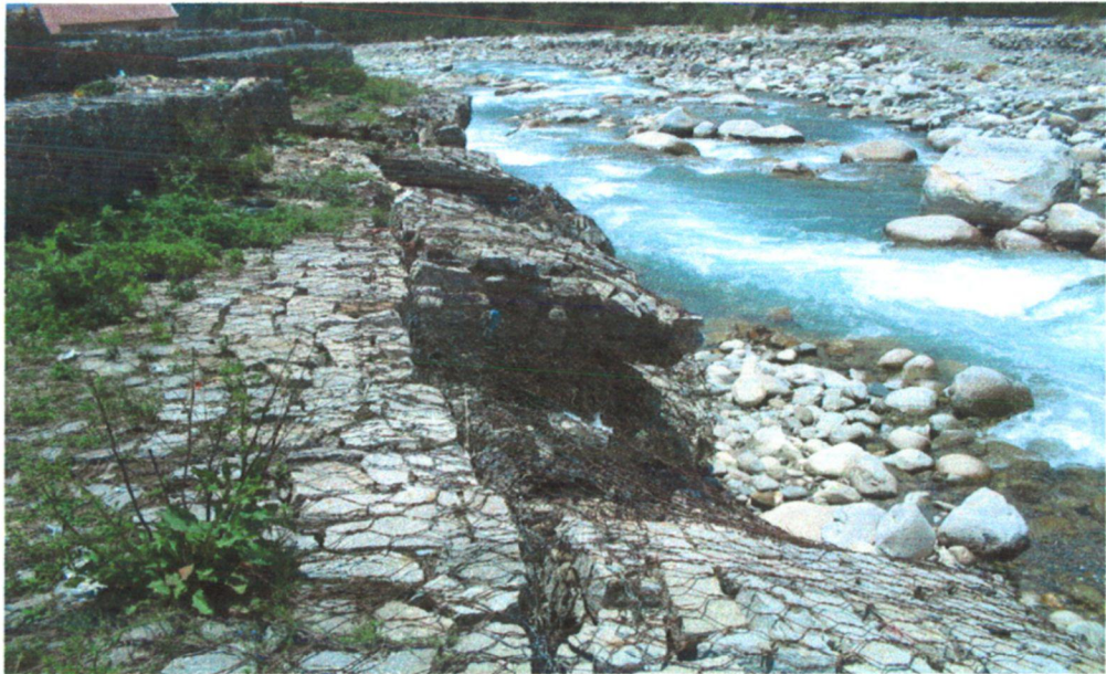
Fig-9.4 Stones are Coming out due to Damage of Mesh
