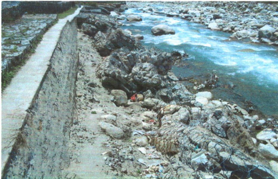
Fig-9.2 GI wire Gabion is affected by Corrosion
