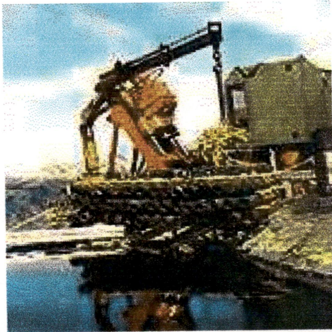
Fig. 4.25 Raiser 170-H drilling 1.5m / 160m water intake shaft 1400m over sea level. (28)
