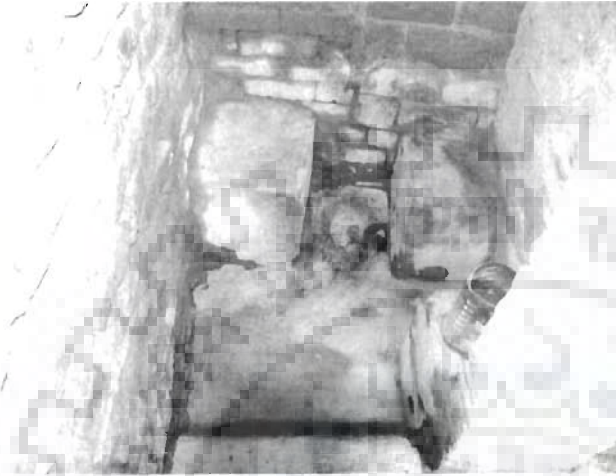
Fig. 5.50 Frontal approach for a dry squat toilet with two cemented platforms to squat.
