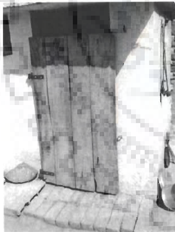
Fig. 5.62 (c) Battered Door of toilet in closed position with no fixtures on outside surface.
