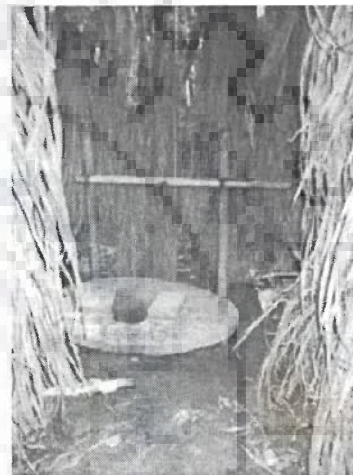
Figure 2.11. Bamboo support poles in a rural latrine in Gobindapur (CRP community project) Source : Jones, H, et al,(2002)
