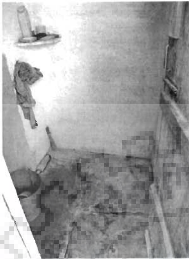
Fig. 5.79 Corner slab to keep soap etc. at 4'0" height in a bathing space.
