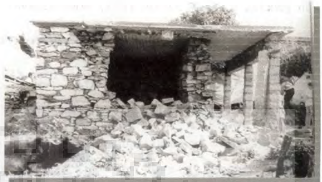
(a) Damage to random rubble stone masonry During Chamoli Earthquake Source: Jain et. al. (1999)
