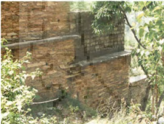
(c) Concrete Block masonry wall constructed over slate and stone masonry wall
