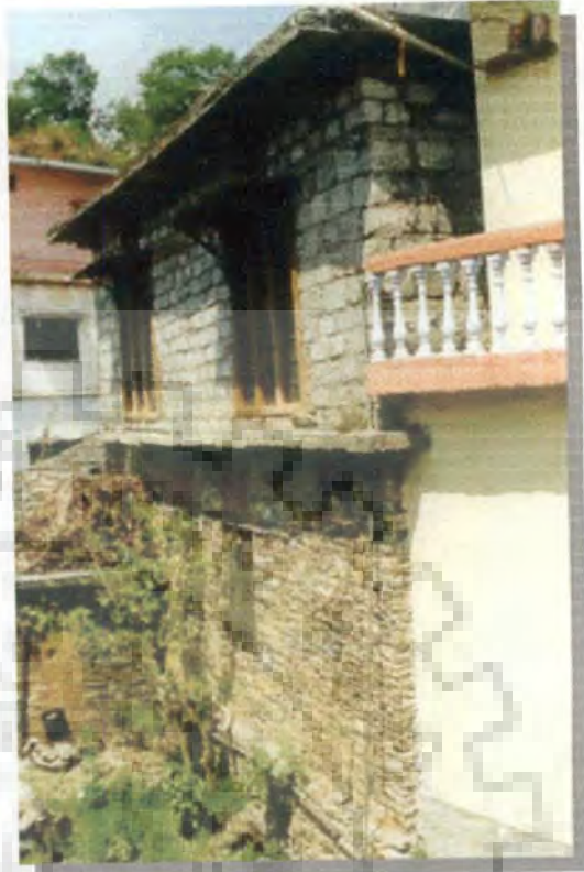
(b) Little Damaged concrete block masonry constructed over stone and slate masonry wall during Chamoli Earthquake Source: Jain et. al. (1999)
