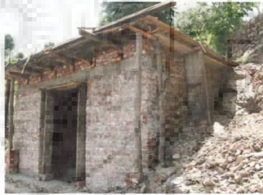
(d) Brick wall being constructed in front side of a stone building
