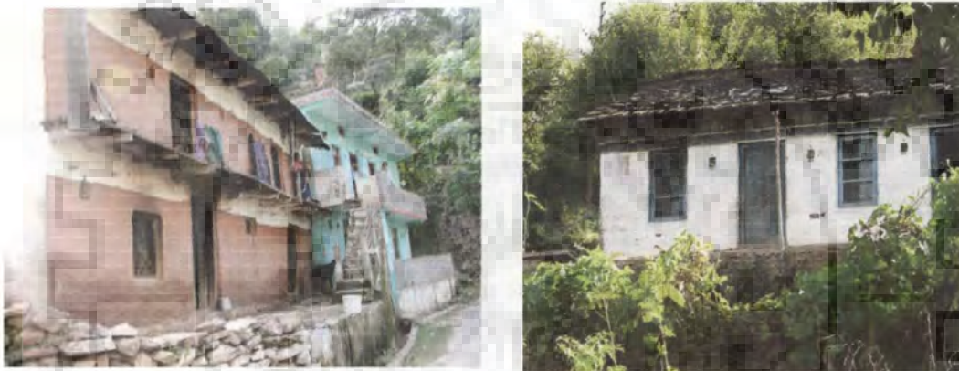
(a) Random rubble stone masonry with mud plaster (b) Random rubble stone masonry with cement plaster
