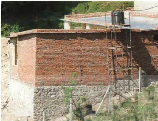
(a) Brick walls without RC frame in Gaja
