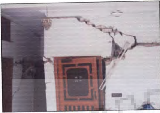
(a) Damaged unreinforced brick masonry wall in Muzaffarabad
