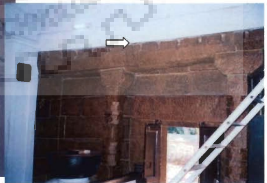
Photo 3.108 Grooves cut over beams, Thiruvithamcode church
