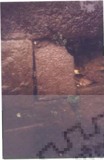
Photo 4.37 Stone slabs with letters used to cover drain in Kottayan Valiya palli
