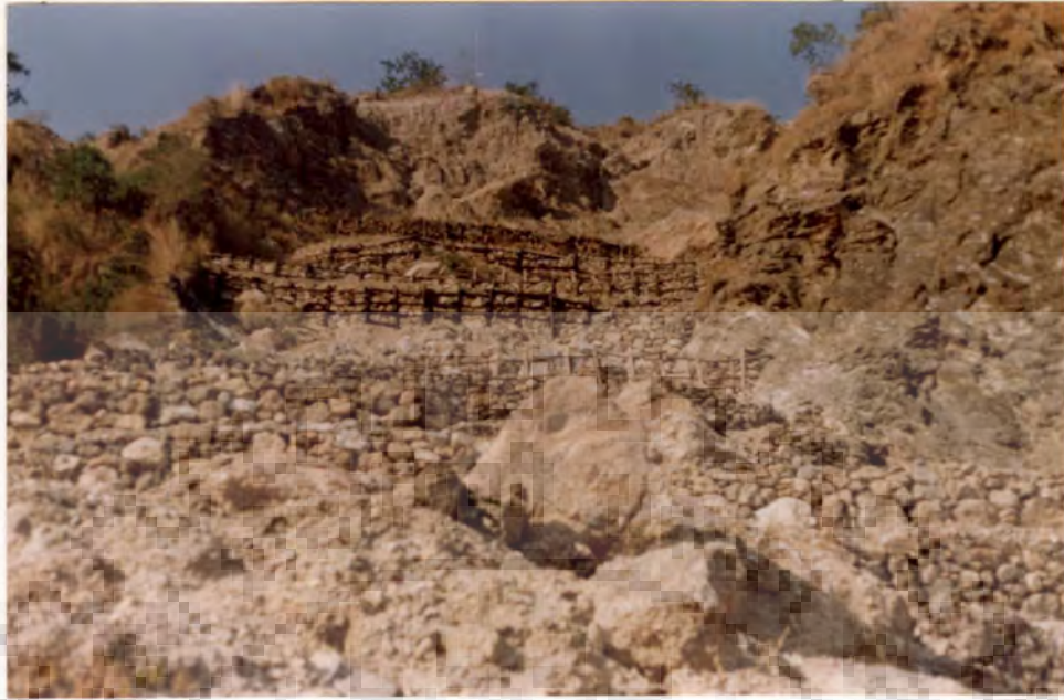
PHOTOGRAPH 3.7- Logwood crib structures filled with stones in the landslide area of Jhandoo-Nala watershed.
