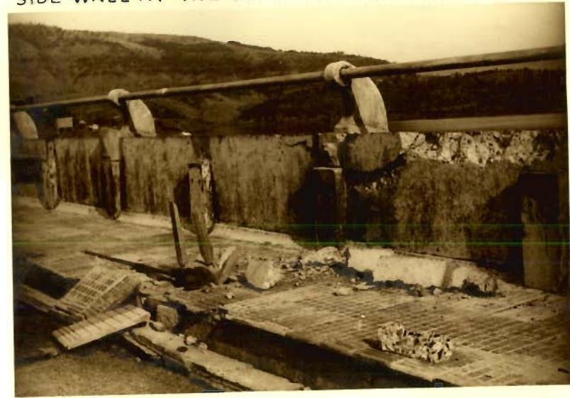
DAMAGED PARAPET WALL AND THE TILES OF THE SIDE WALL AT THE TOP OF THE KOYNA DAM
