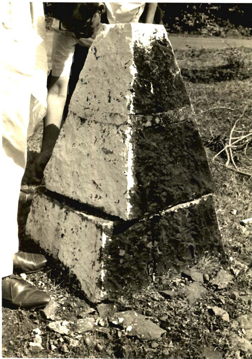
Figure 41. Rotational movement registered on a pillar on Helwak Chiplun road-Near Dondchiwadi
