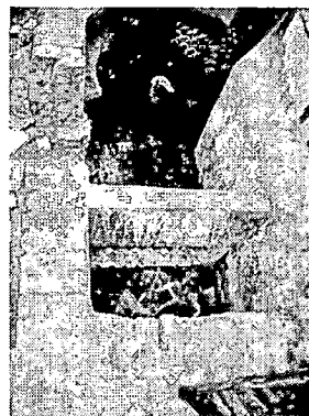
Figure 5.7.6.5 Drains falling into sewer which is clogged (Source: By Author)
