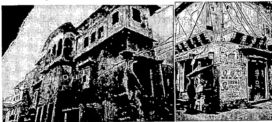
Figure 3.4.4 Deteriorating condition of heritage buildings
