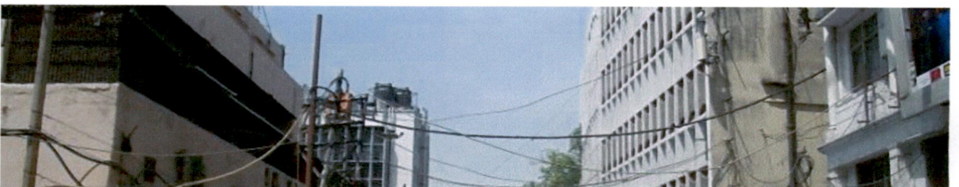
Figure 117 Cluttered overhead wires
