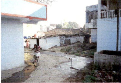
figure 5.13 Dilapidated house at a prime location of former village which is fast changing its character in wake of urbanization, the house is in bad shape will soon be replaced by the force of land economics
