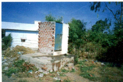
figure 5.4 The figure shows the condition of soak pit latrine of a village residence the important
