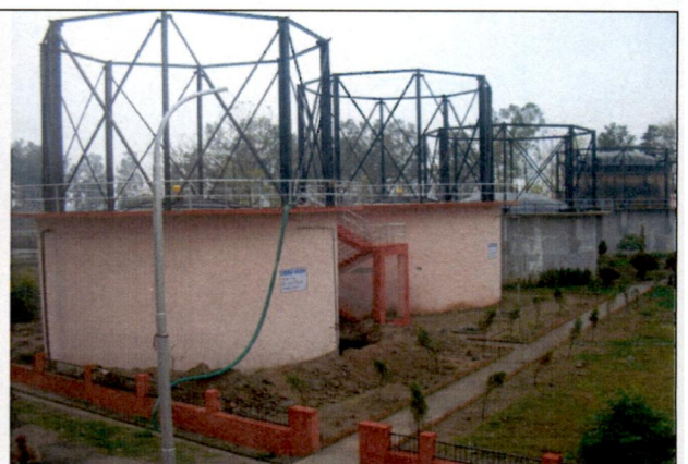
Fig 4.3.6: Bio Gas Tanks
