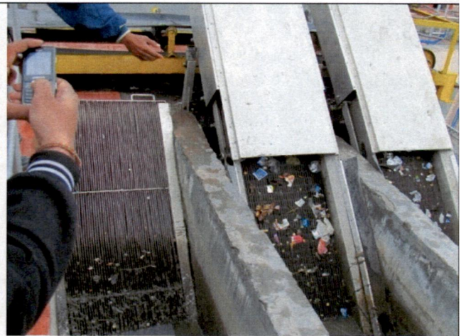
Fig 4.3.2: Mechanical Grit Chamber
