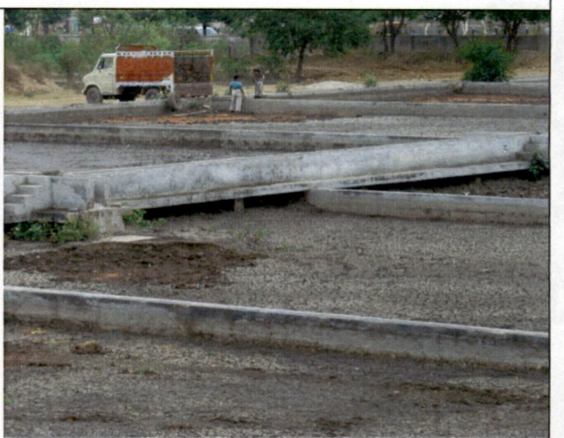
Fig 4.4.6: Sludge drying bed
