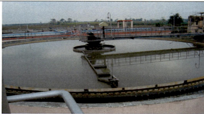
Fig 4.3.3 Primary Settling Tank
