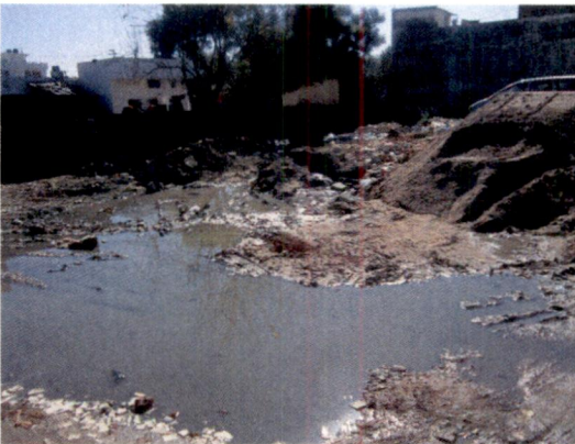
Figure 3.17: Sewer line is very old and choked.
