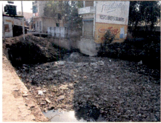
Figure 3.16: Solid waste in sewer line.
