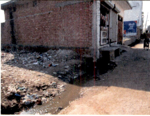
Figure 3.15: Sewage flow is draining through the surface.
