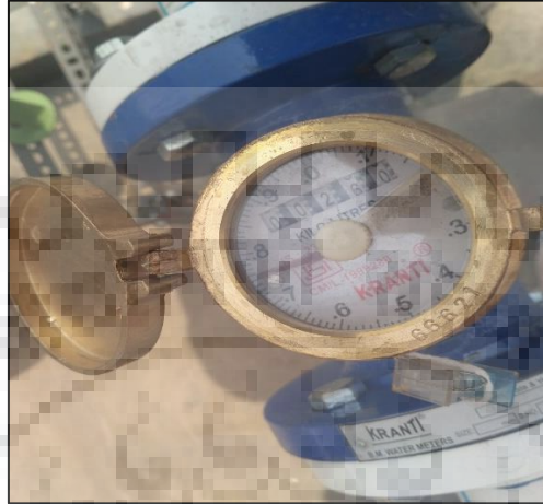
Figure 3.7 Water flow meter
