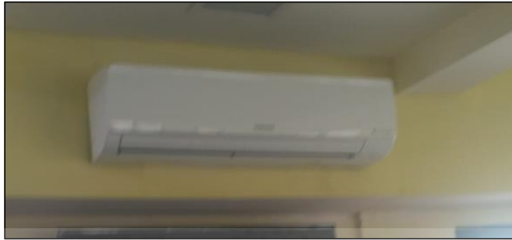
Figure 3.3 Indoor HVAC unit
