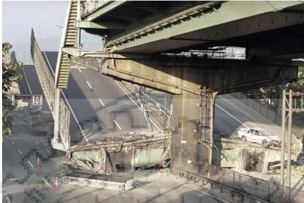
Fig. 1.4 Failure of Nishinomiya-Ko bridge during 1995 the Great Hanshin-Awaji Earthquake
