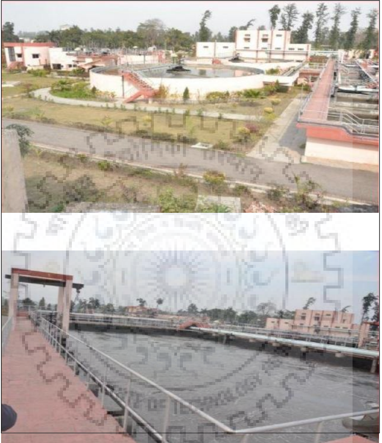
Fig 2.2 27 Mld sewage treatment plant JagjeetpurHaridwar(27)
