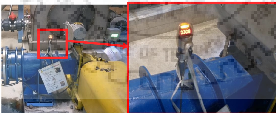
Figure 6.14 GP-M pressure sensor fixed on penstock
