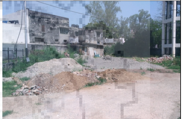
26. Excess construction material lying.
