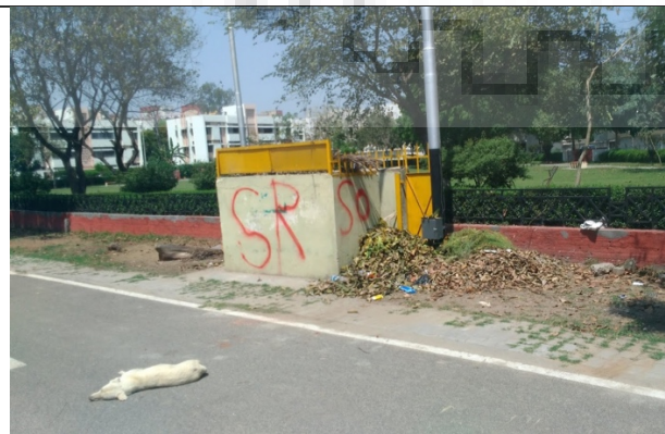
9. Damaged door lock
