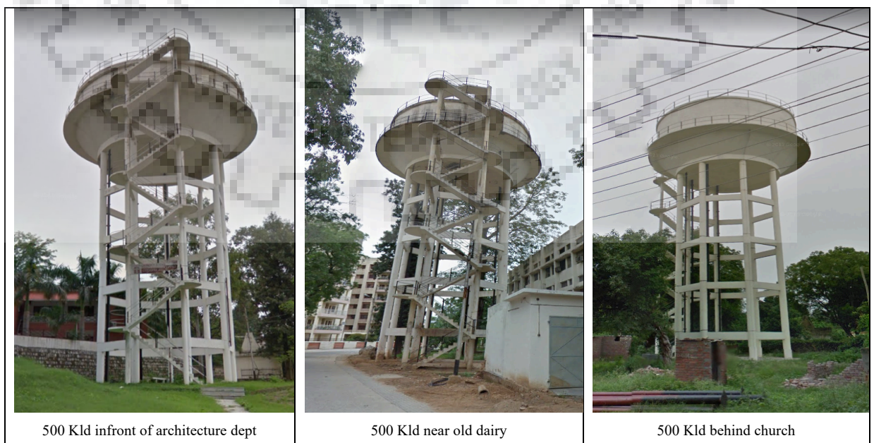
Fig -2.5 Water tanks within campus
