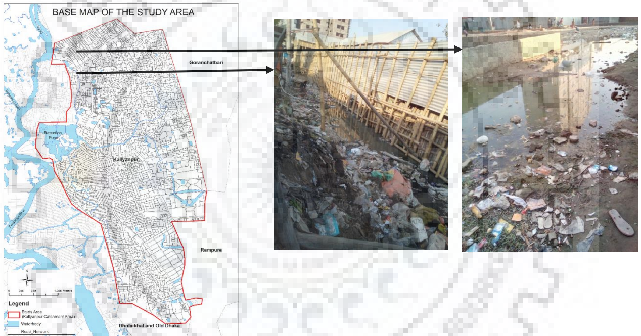
Figure 43 Poor Condition of Drainage Facility in Study Area
