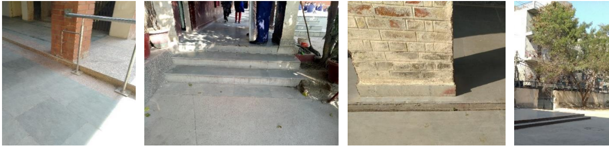
Figure 39 Lack of Attention to details _ Barriers
