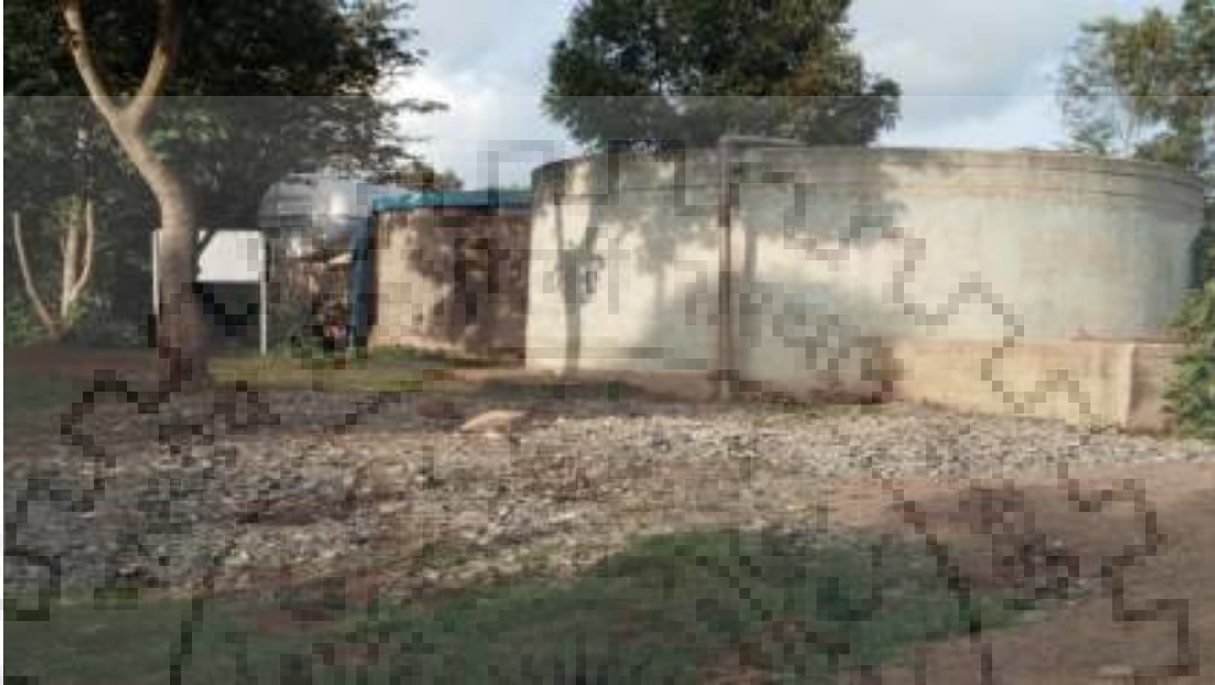
APPENDIX A1 KMG water tank
