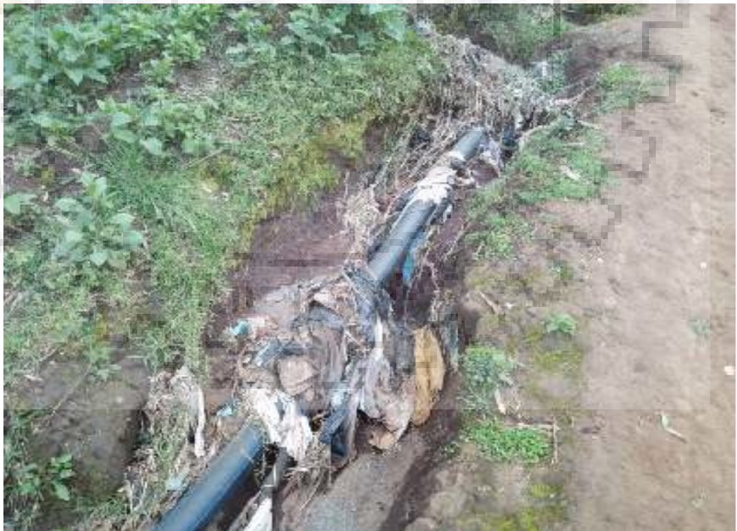
APPENDIX A5 Erosion effect on pipes
