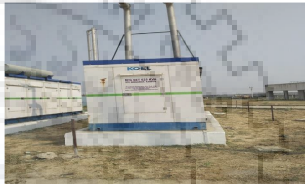
Fig.3.4.2d Dual Fuel Engine at STP plant
