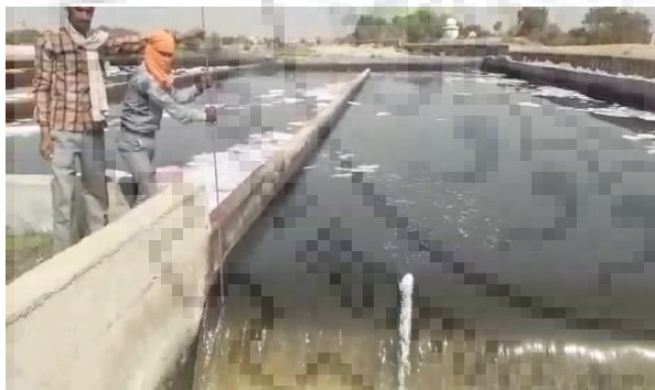
Fig.3.4.2e Treated effluent falling into outlet C/h
