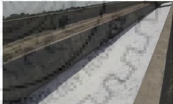
Fig.3.4.2f Outlet channel of STP Plant
