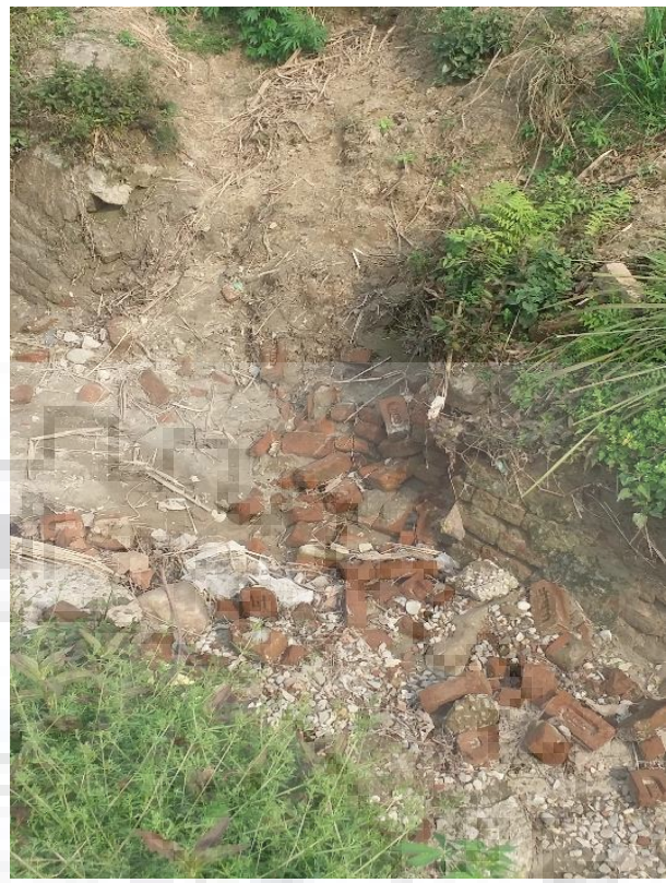
Photo 5.6 Damaged lining wall – (b)
