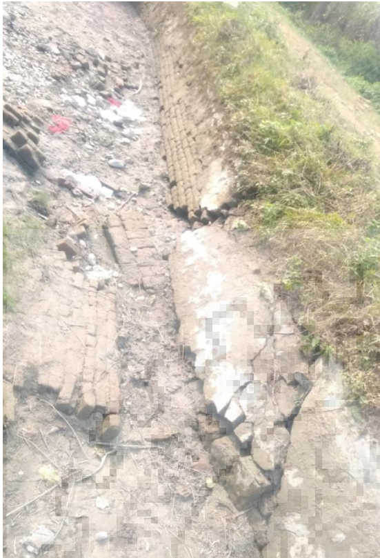
Photo 5.5 Damaged lining wall – (a)
