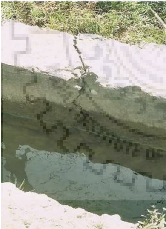
Photo 5.11 Cracks in lining
