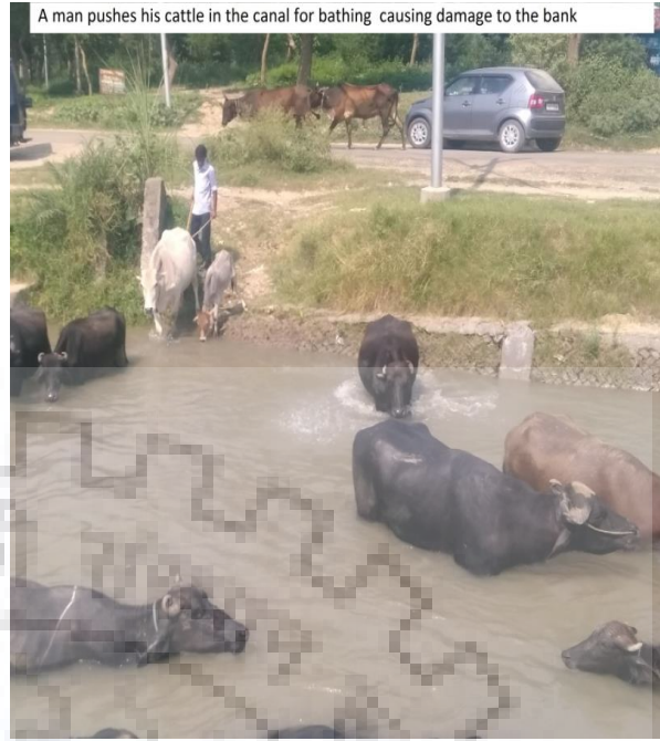
Photo 6.4 Social factors damaging canal lining
