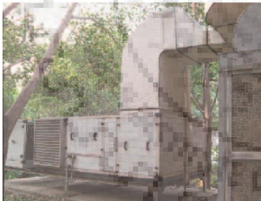
Figure 41 Prototype Air- Handling unit
