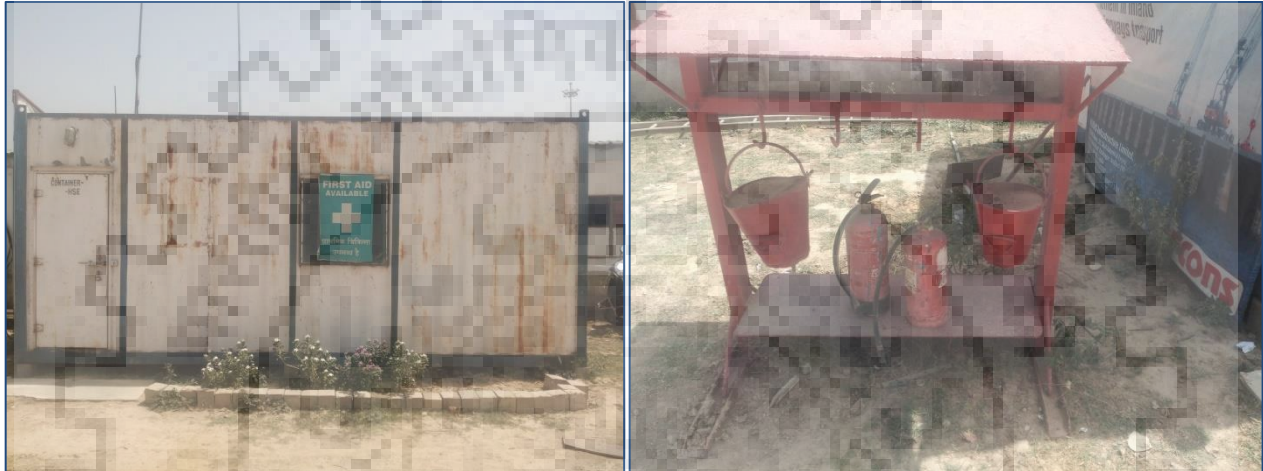
Figure 18: Safety equipment at Varanasi inland waterway terminal
