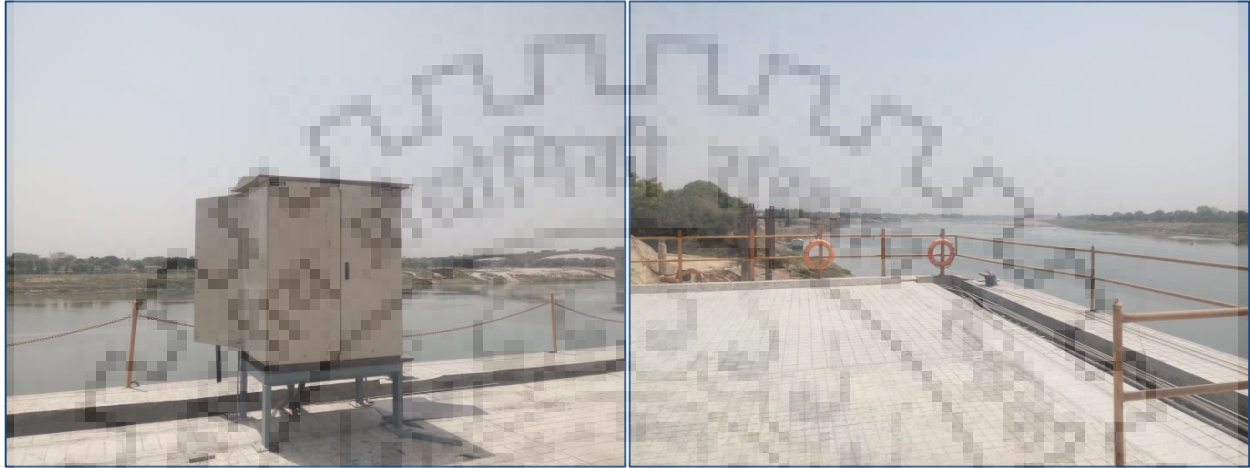
Figure 20: Missing warning signs at Varanasi inland waterway terminal
