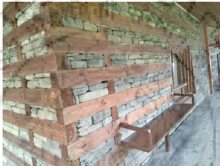
Figure 1 Corner construction detail of kath-kuni style housing. The timber bands run along both sides of the wall and are connected by pins along their length, and at the corners.
